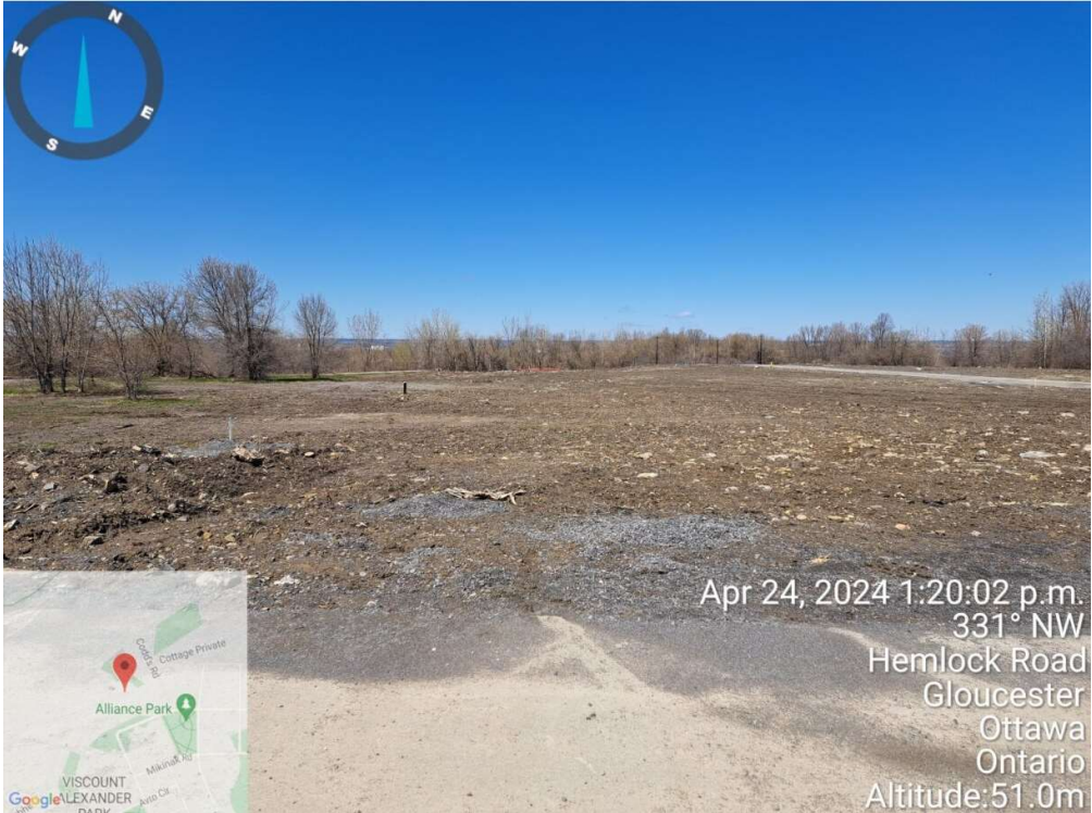
Standing at southeast side of Street No.1 and Looking towards northwest of Block 6 : No indications of existing slope greater or equal to 2 m in height or any settlement.
