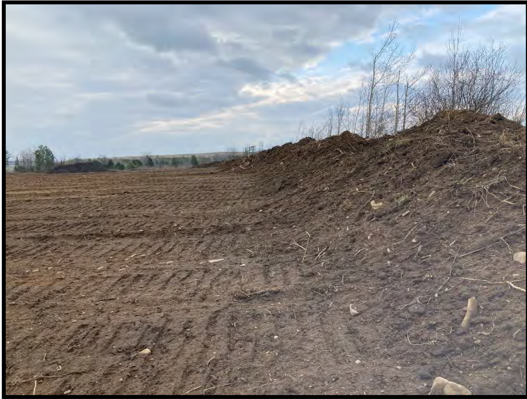
Figure 11: View of stockpiled soil along boundary of study area, bulldozer tracks. (MH1174-D033)
