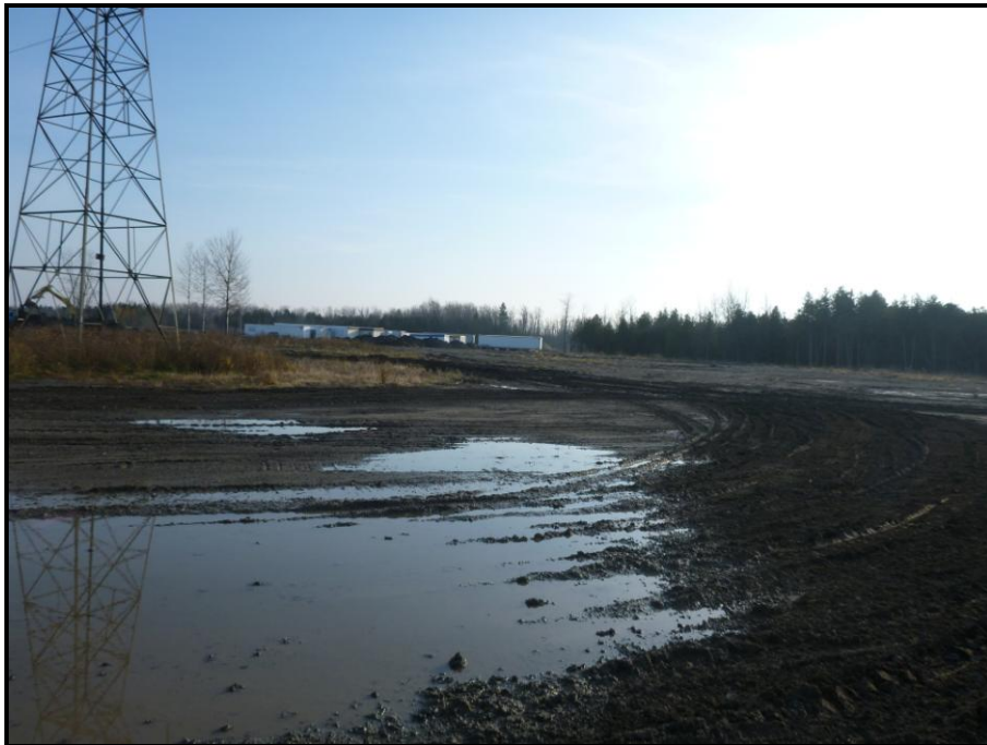
Image 10. View of levelling fill in the western end of the property, facing south. (PR16-42D041) Note the piles of imported topsoil in the distance (in front of the white trailers).
