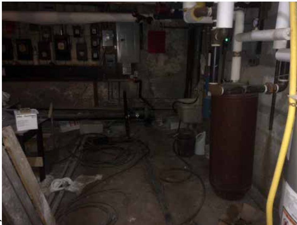
Photograph 12. View of the mechanical room, located in the basement of the church
