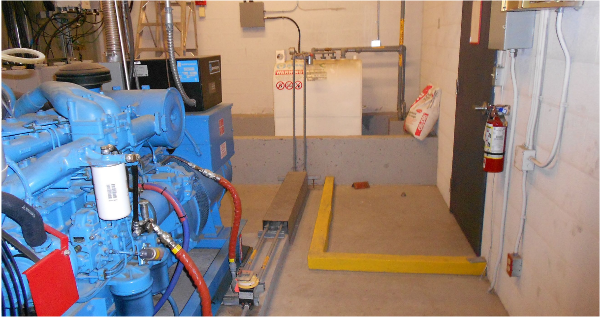
Photo 19 View of diesel generator and day tank located in penthouse of Tower 3.
