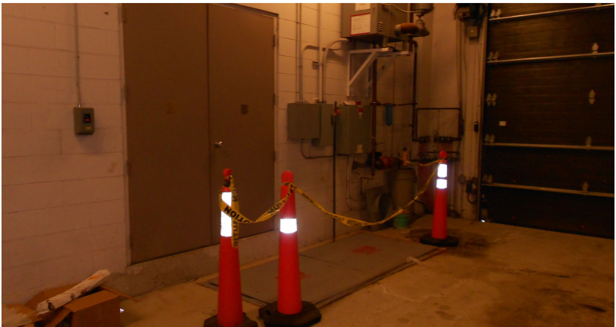
Photo 22 View of sump pump pits and glycol system for Tower 2 basement loading ramp with trench drain.
