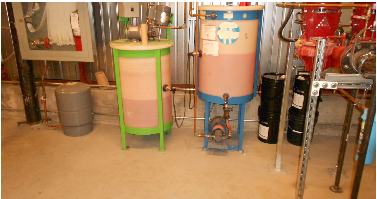
Photo 24 Typical penthouse glycol loop system and reservoir tanks.
