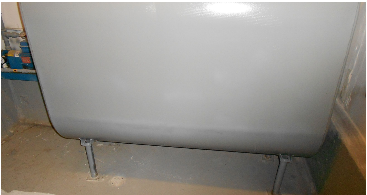
Photo 20 View of bulk diesel tank on ground floor of Tower 3 (feeds day tank located in Tower 3 penthouse).
