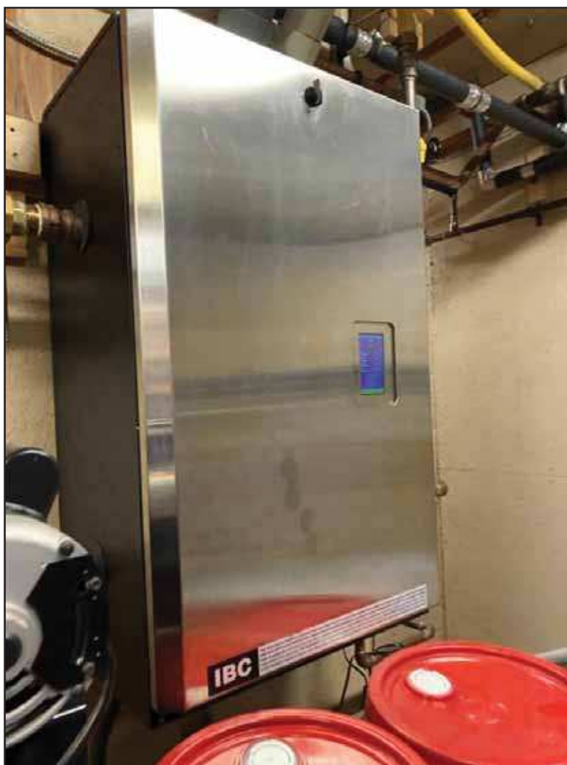
Photograph 13: View of car wash heating system.
