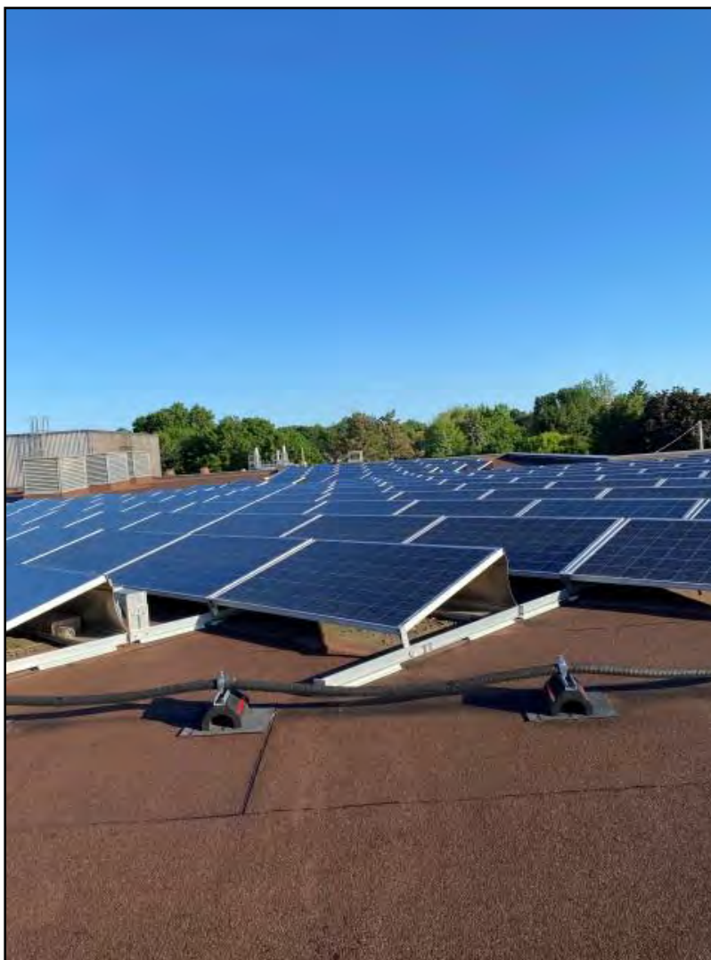
Photograph 20: View of rooftop solar panels.
