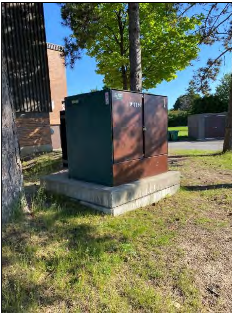
Photograph 7: View of a ground mounted transformer on the exterior south-east corner of the subject building.
