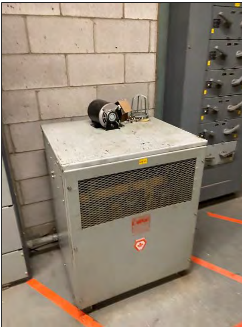
Photograph 30: View of a transformer in mechanical room 222.
