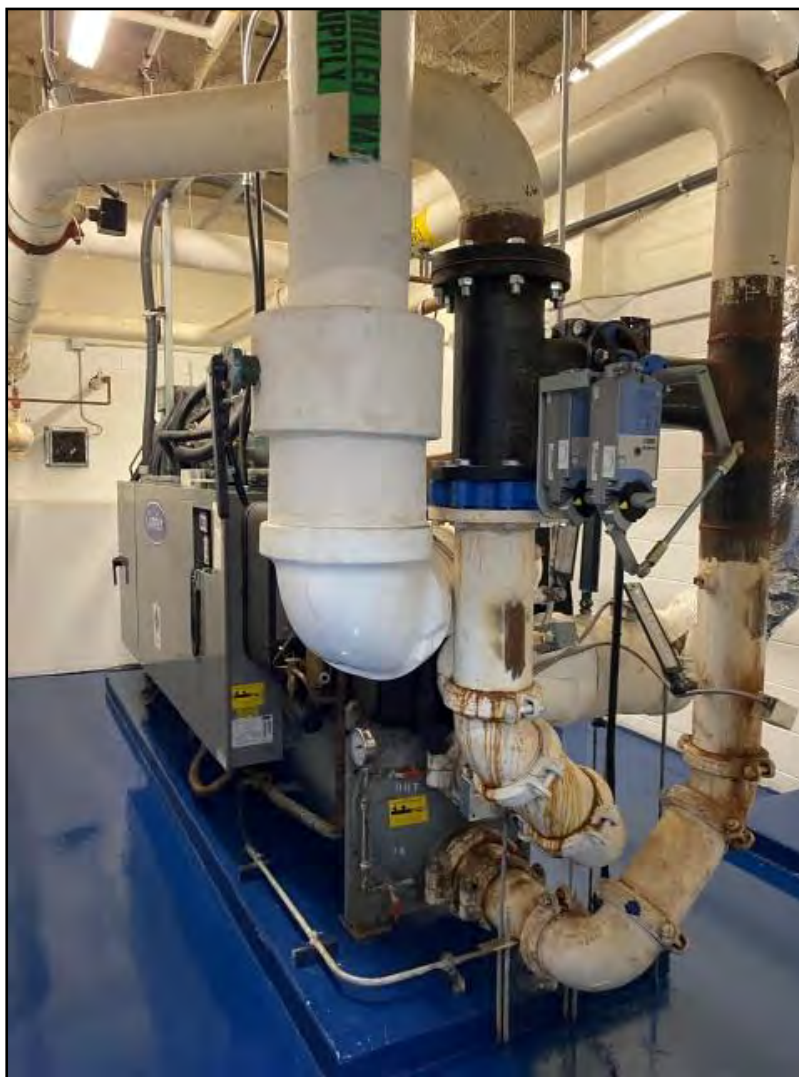
Photograph 18: View of a refrigeration unit in mechanical room 241b.
