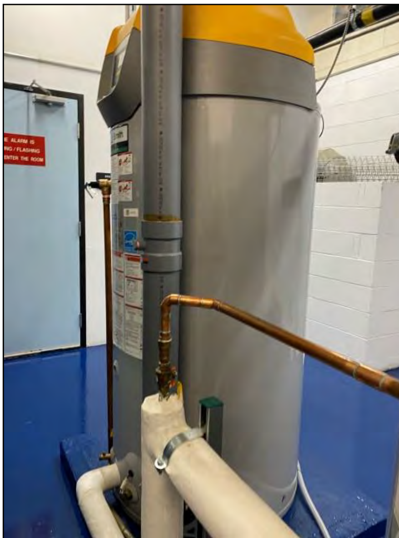
Photograph 14: View of a hot water heater in mechanical room 241.
