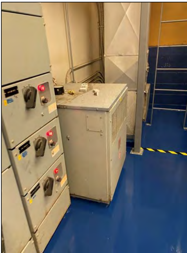
Photograph 32: View of a transformer in mechanical room 238.
