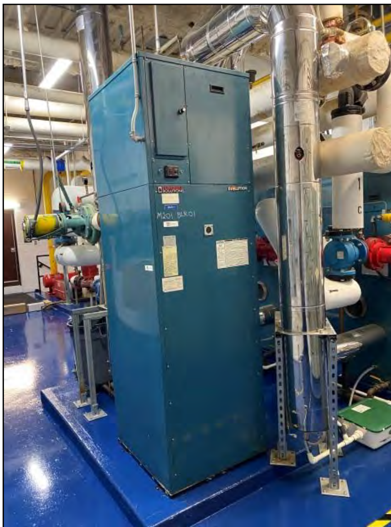
Photograph 13: View of a gas fired boiler in mechanical room 241.
