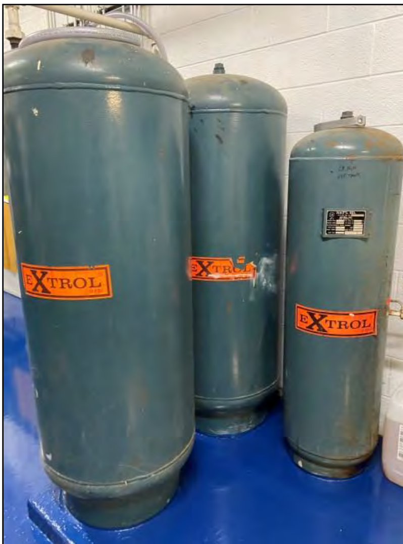
Photograph 16: View of expansion tanks in mechanical room 241.
