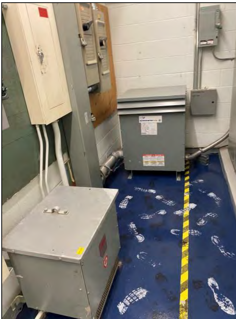
Photograph 25: View of a transformer in electrical room 140e.
