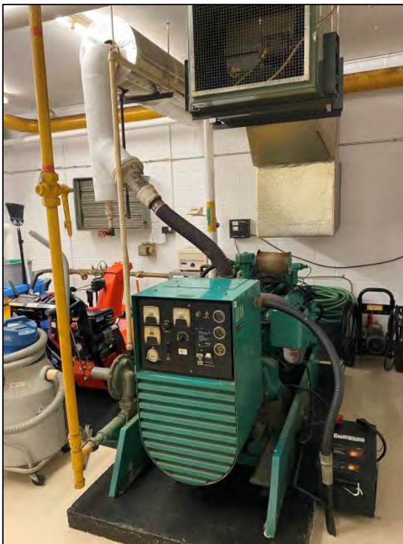
Photograph 26: View of a natural gas fired generator in room 140f.
