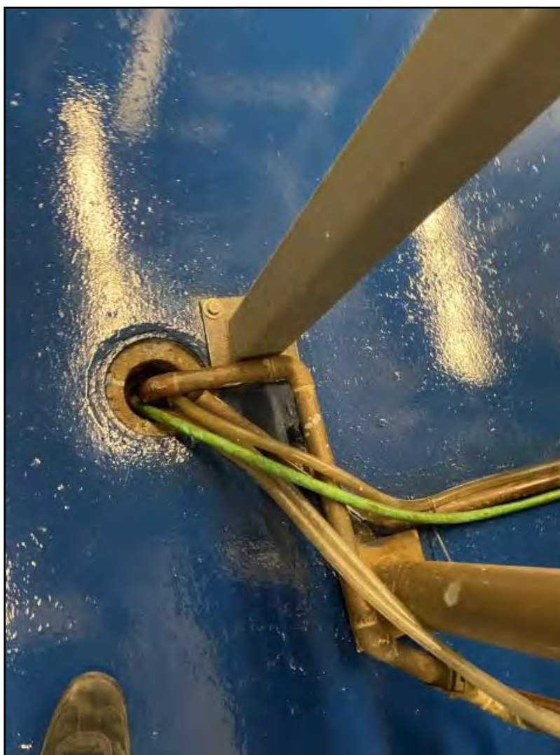
Photograph 31: View of a floor drain in mechanical room 238.
