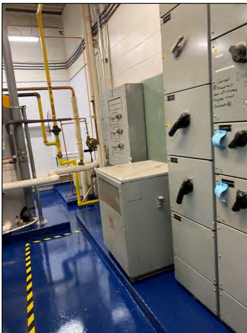
Photograph 22: View of a transformer in mechanical room 241.
