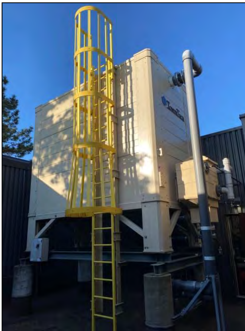
Photograph 19: View of a cooling tower in mechanical room 241a (lower roof).
