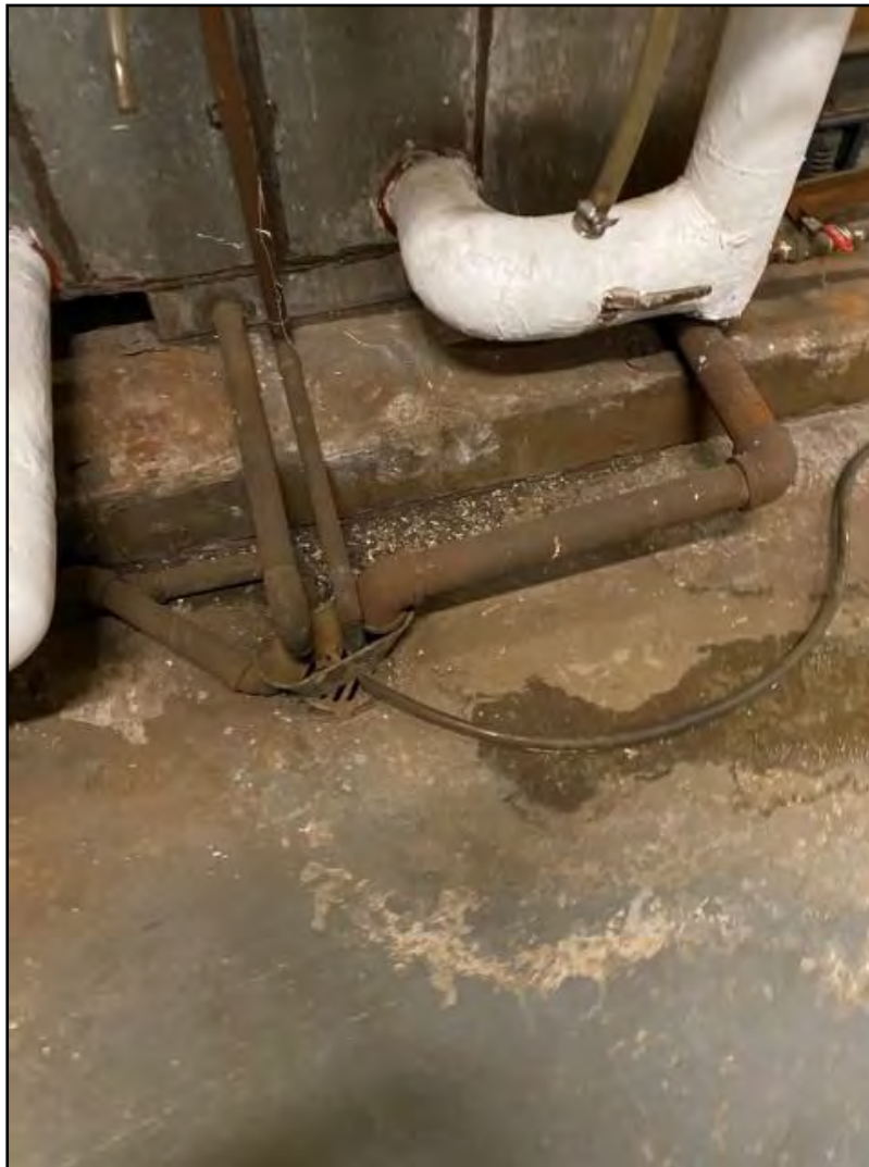
Photograph 29: View of a floor drain in mechanical room 222. Minor rust, dirt, and water staining present.
