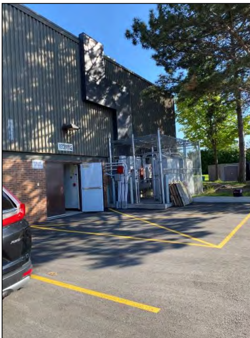
Photograph 10: View of an electrical area on the south side of the building. Presumed battery storage location for rooftop solar panels.
