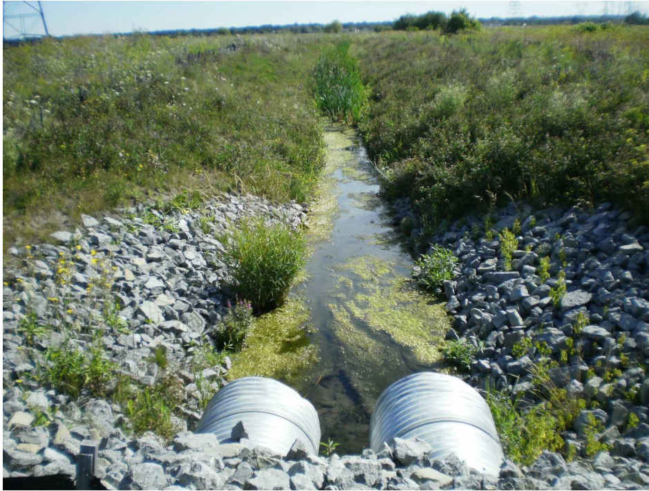
Photo 1 – Realigned portion of the West Tributary downstream of the new high school. View looking east
