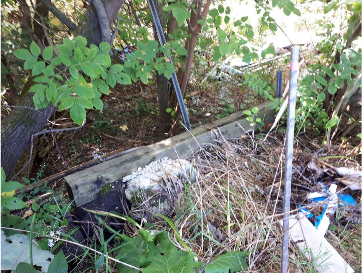
Photograph No. 19: Homemade retaining wall with signposts and 6x6 lumber at crest of slope, section B-B
