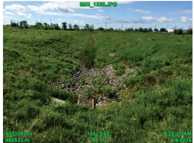
Photo 8 – Reach 2 looking upstream at Innes Road – note Reach 2 is piped downstream of this location
