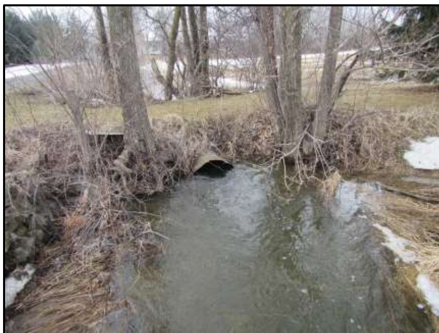
Photograph 4: Survey Site #1 - 60 cm CSP culvert under the driveway west of March Road (facing upstream) (March 30 th , 2018).
