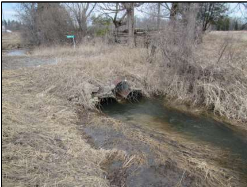
Photograph 2: Survey Site #1 - Three (3) stacked 60 cm CSP culverts under the old farm driveway, east of March Road (facing upstream) (March 30 th , 2018).
