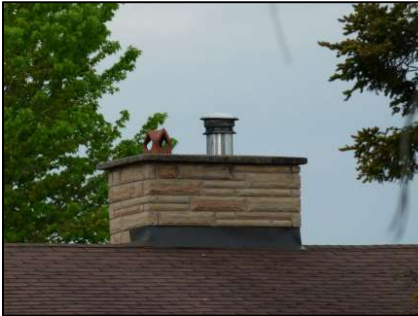
Photograph 31: Chimney at 1015 March Road. Note metal cap and ceramic liner (May 24 th , 2017).
