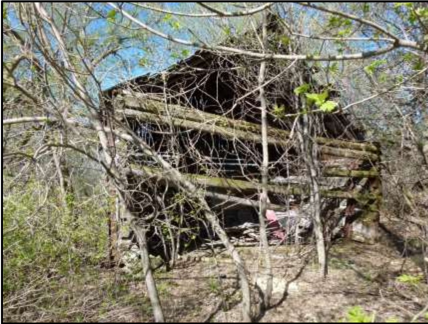
Photograph 47: Building #6 – Looking west at the collapsing barn (May 8 th , 2018).
