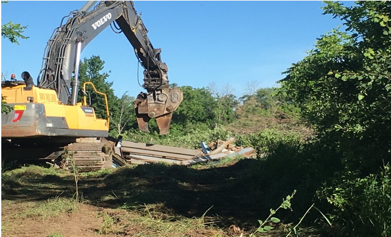
Photograph 5: Photograph illustrates removal of scrap metal northeast of residential dwelling, facing north.
