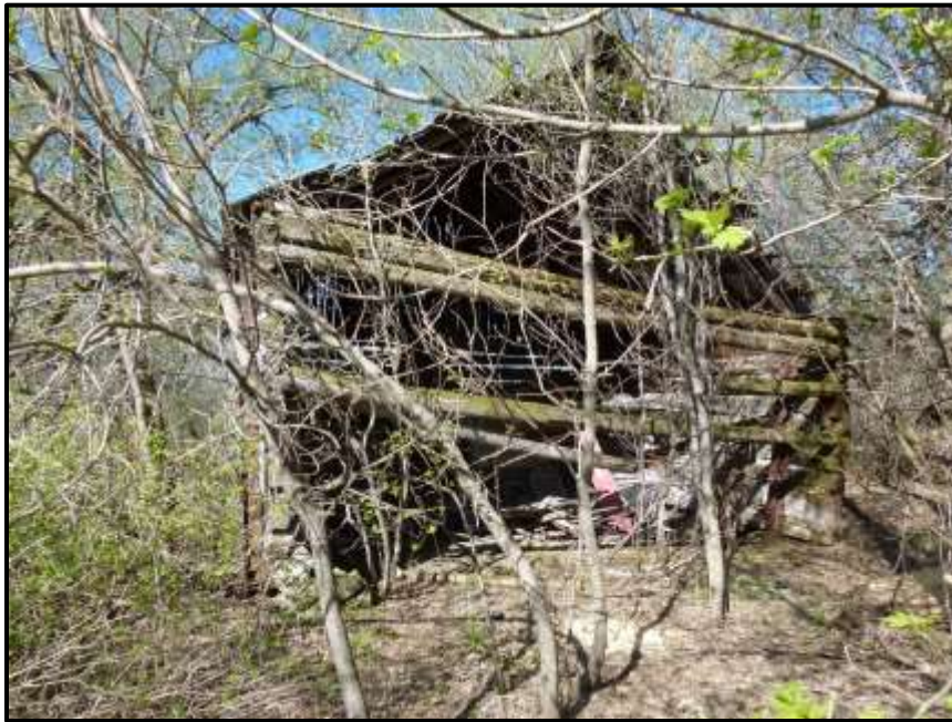
Photograph 48: Building #6 – Looking west at the collapsing barn (May 8 th , 2018).
