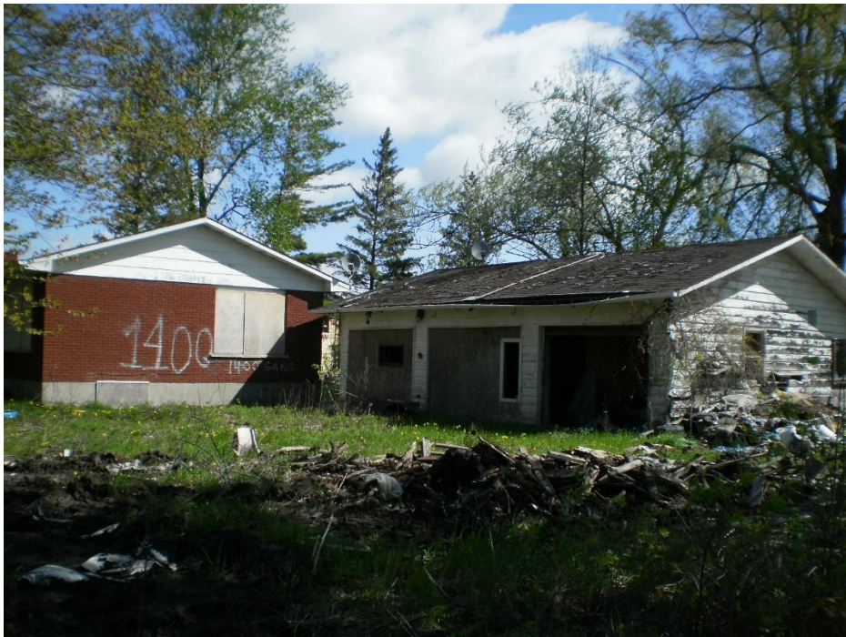
Photo 6 – Boarded up residence and garage with open doors in the northwest portion of the site. View looking northeast
