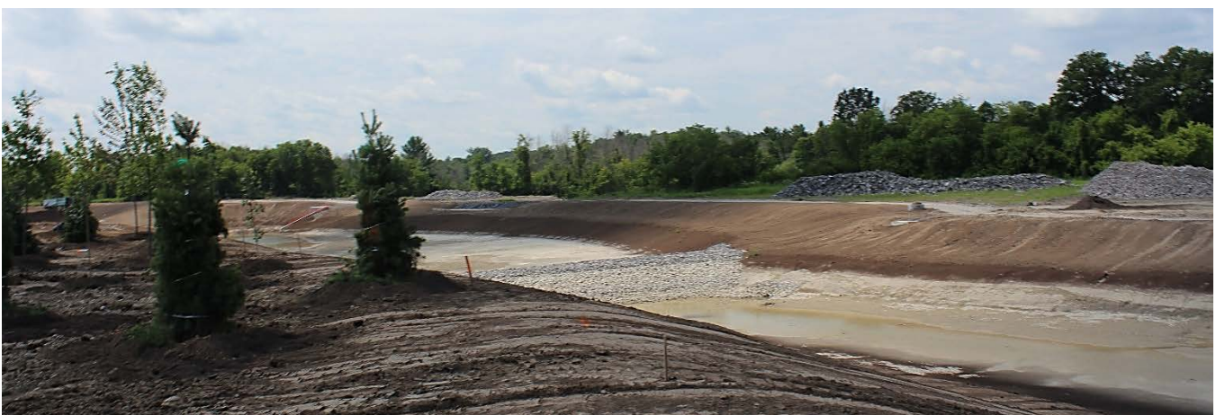
Figure 10: View south from 750 River Road of the stormwater management pond under construction.
