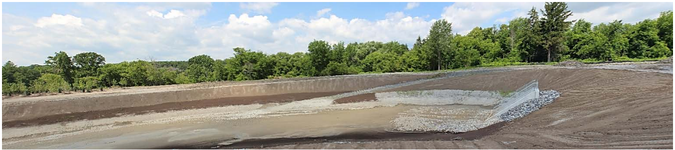
Figure 23: View northwest of part of the stormwater management pond on 750 River Road.
