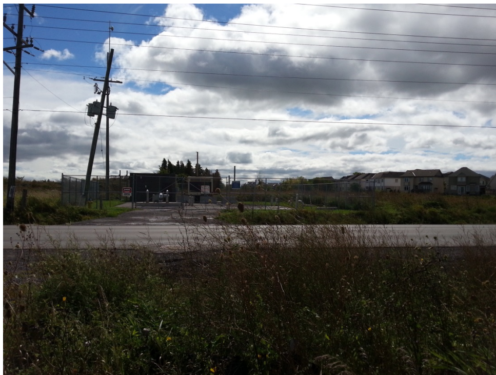
Photograph 3: Looking south at pole mounted transformers and the Maple Grove Road pumping station.
