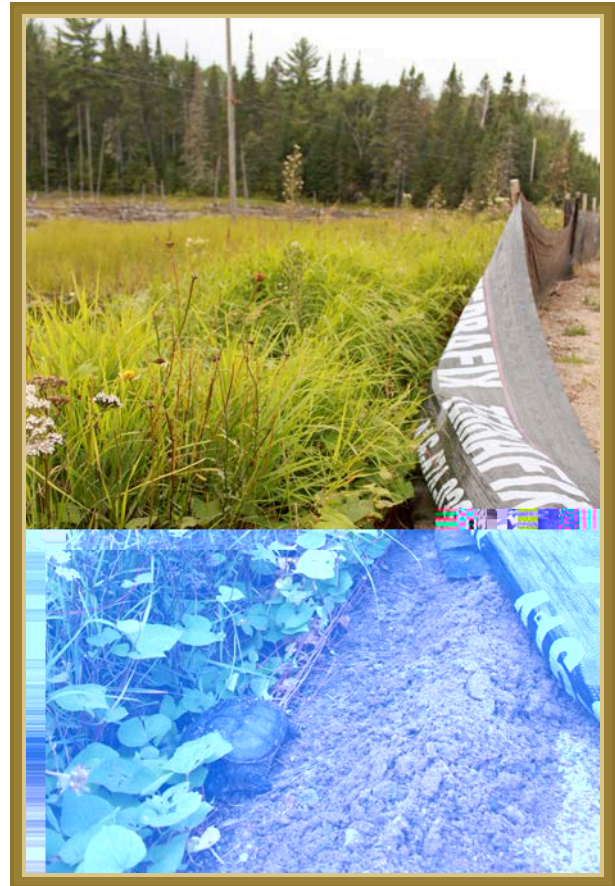
Plate 1. Light-duty geotextile fencing with pre-attached wooden stakes used to exclude turtles from a road as seen on a regular maintenance check (photo credit: Brad Steinberg).
