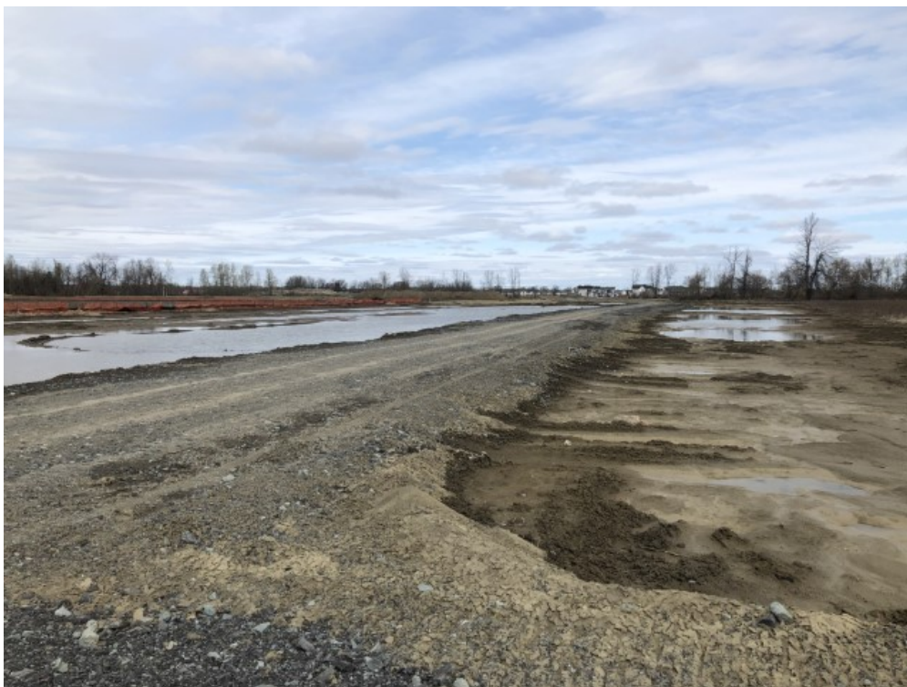
Photo 4: Looking northwest at the residential development occurring on the adjacent lands west of the Site includes the fill piles and standing water.
