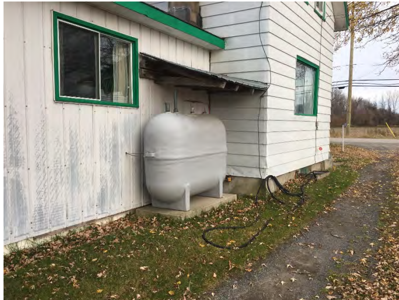
Photo 2 – View of the heating oil AST located along the exterior of the western wall of the house on the 6409 Perth Street portion of the Site.
