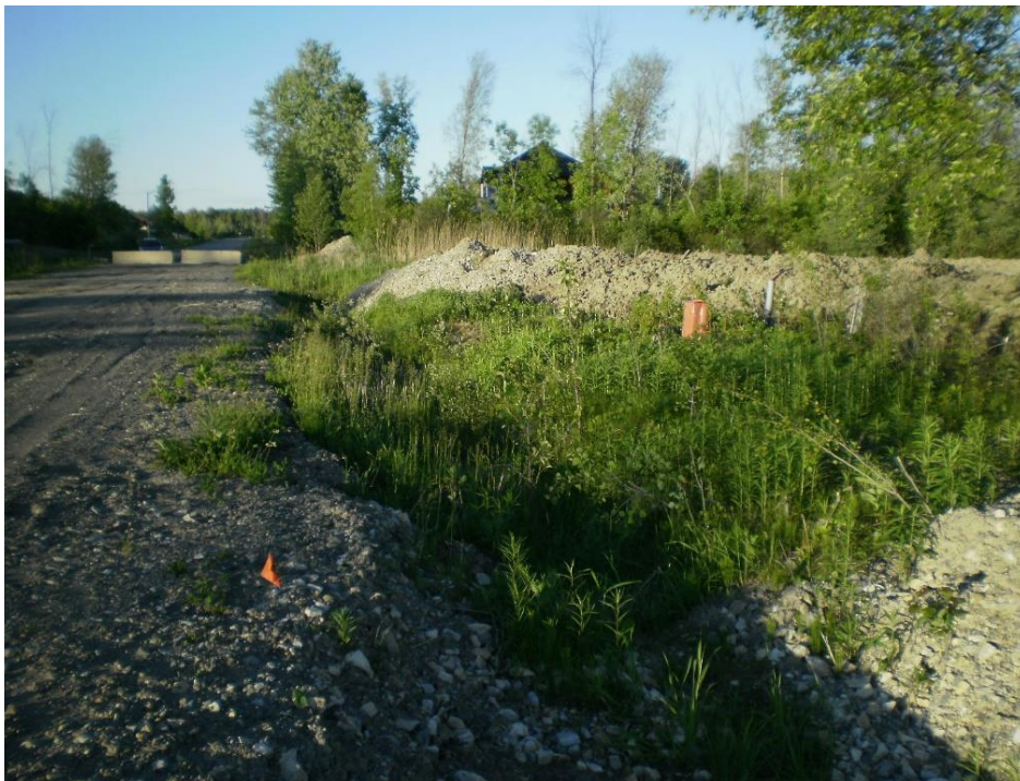
Photo 6 – Dry ditch along the south side of the Tullamore Street extension. View looking east, with Phase 2 houses in the background
