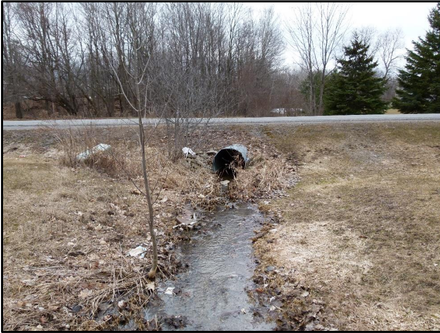
Photograph 11: Looking upstream at the 75 cm CSP culvert under Marchbrook Circle (April 4 th , 2022).
