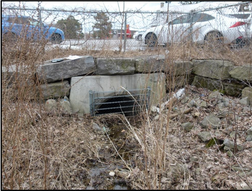
Photograph 1: Looking downstream at the 1.3 m wide concrete pipe under March Road (April 4 th , 2022).
