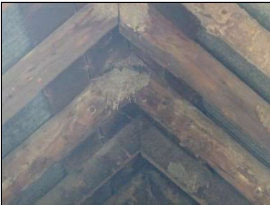
Photograph 23: Active Barn Swallow nest (center) and inactive Barn Swallow nest (right) within the collapsing barn (May 12 th , 2018).
