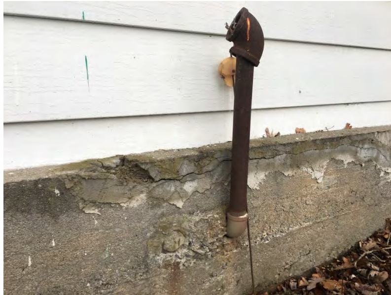
Photo 3 – Piping assumed to be from old fuel oil AST in the basement. Observed along the north wall of the house.
