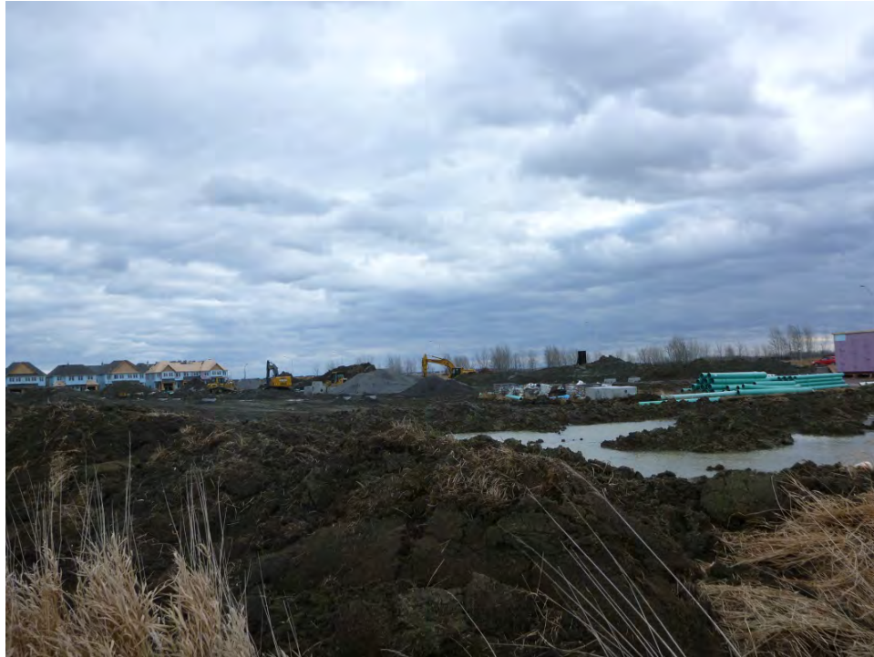
Image 17: Land development being undertaken in the southeastern portion of the property, looking east.
