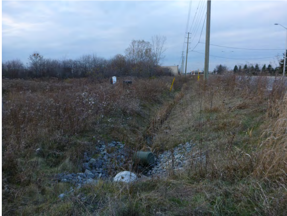
Image 15: Drainage ditch west along Mer Bleue Road causing deep ground impact. Photo taken looking northwest.
