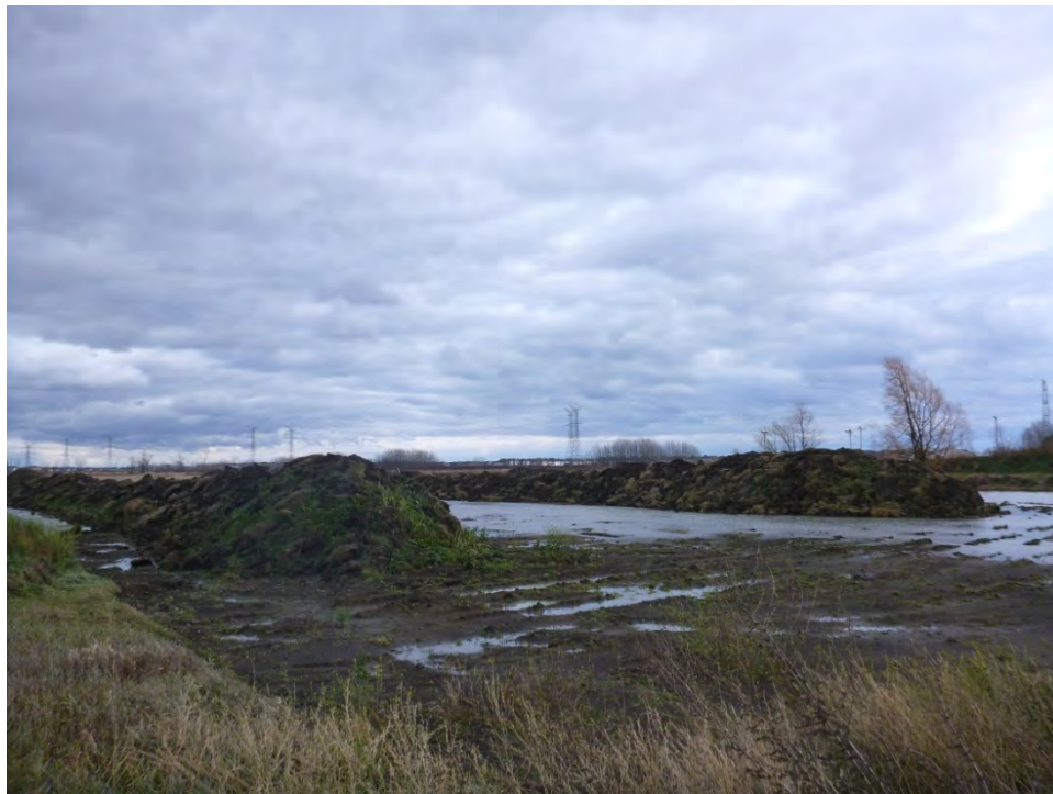
Image 16: Significant soil stripping and deposits northeast along Mer Bleue Road, facing east.
