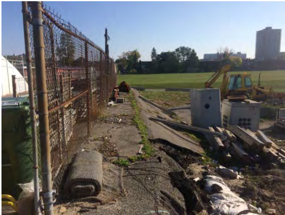
Photo 4: Debris in storage area of 933 Gladstone, facing east.
