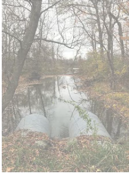
Photo 5 – Discharge pipes into river tributary on the south-east corner of the Site at 3305 Borrisokane Rd
