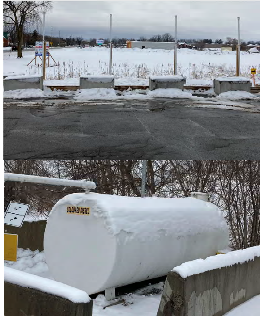
Photograph 11 – Above-ground and below-ground fuel storage tanks at the gas station approximately 75 meters south of the Site.
