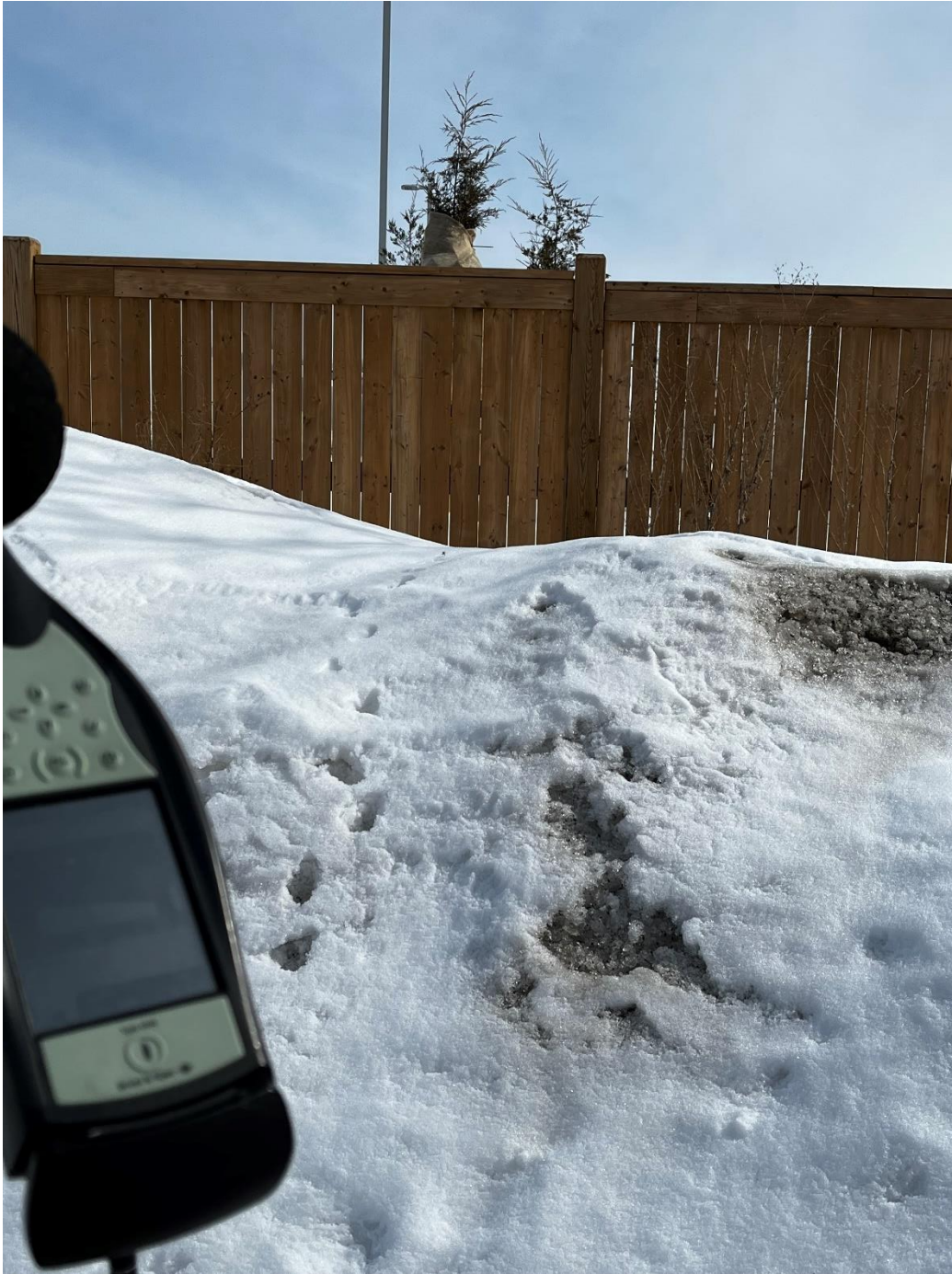
PHOTOGRAPH 5: EXISTING PERIMETER FENCE GAPS BETWEEN WOOD PLANKS
