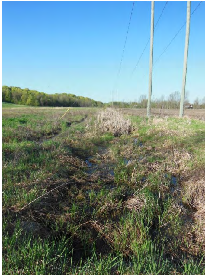
Figure 101: Permanently wet area in Operation 16 at base of slope (D271).
