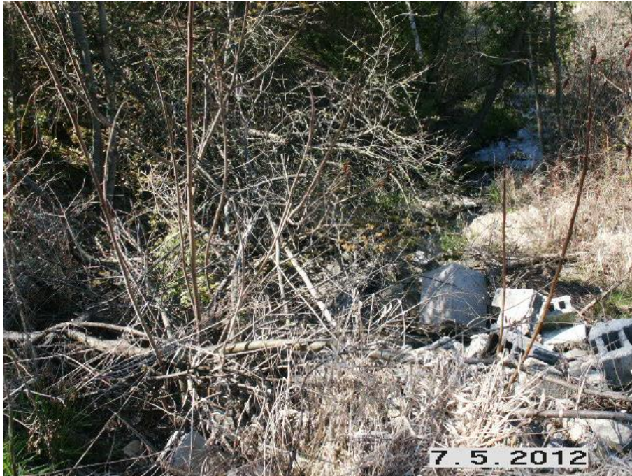
Photo 4 – Culverts and other debris impact the connectivity of the south tributary downstream (west) of the site. View looking west
