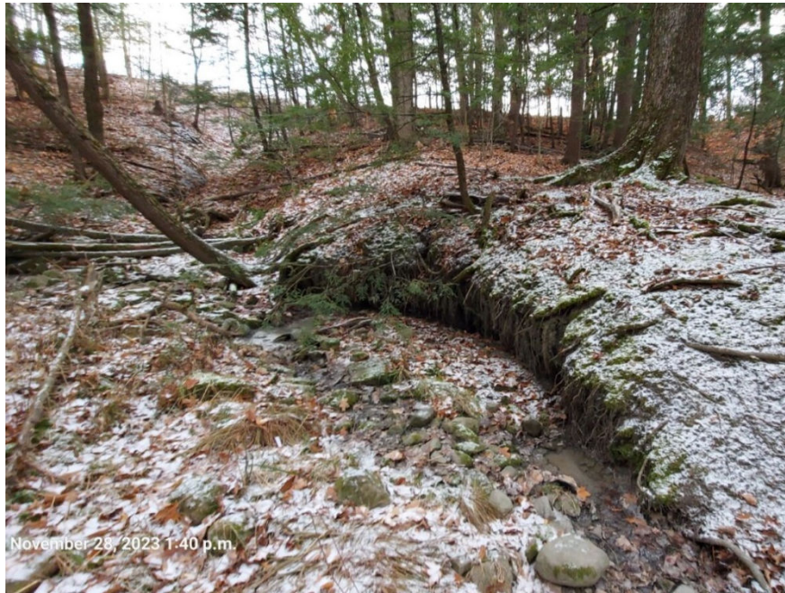
Photograph taken facing upstream along T2 . Undercutting, exposed roots and rotational slumps were commonly observed.
