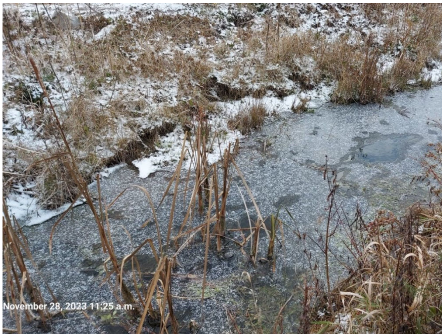
Photograph taken facing the left bank at the downstream extent of R1 . Minor scour was observed along both banks.
