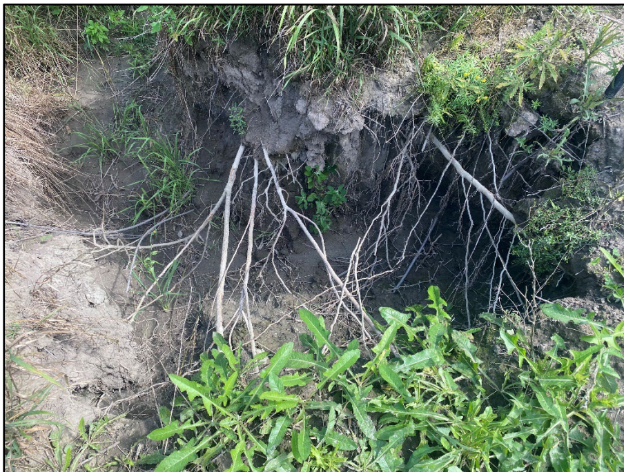
16. Mud Creek– Drainage from the adjacent field has resulted in a significant washout along the southern bank of Mud Creek
