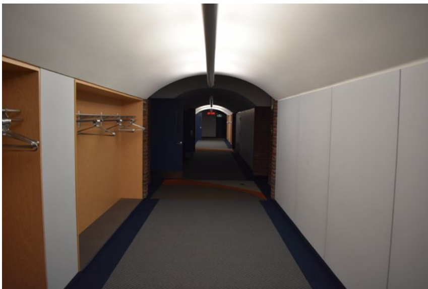
Figure 27. Material finishes in some areas of Building J have been replaced relatively recently (ERA, 2021).
