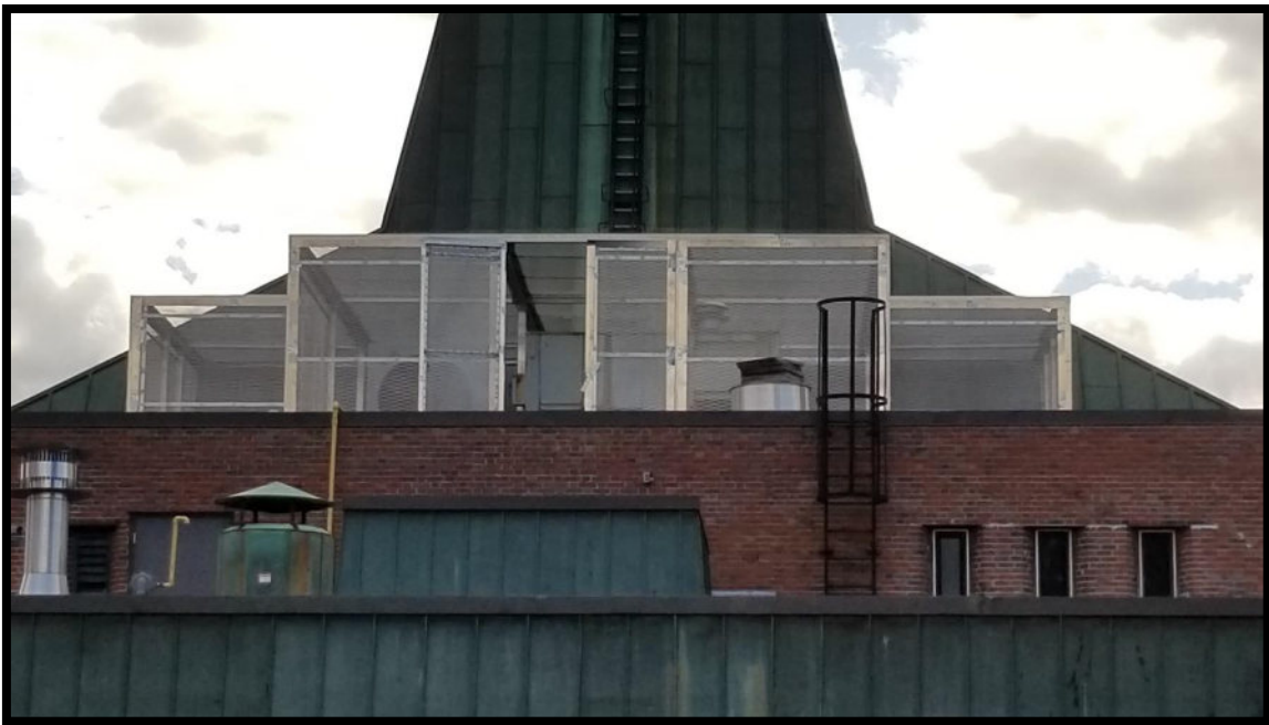
Photograph 4: View of the rear of Building A of the Site, facing south. Rooftop mechanical equipment is present on top of the building.
