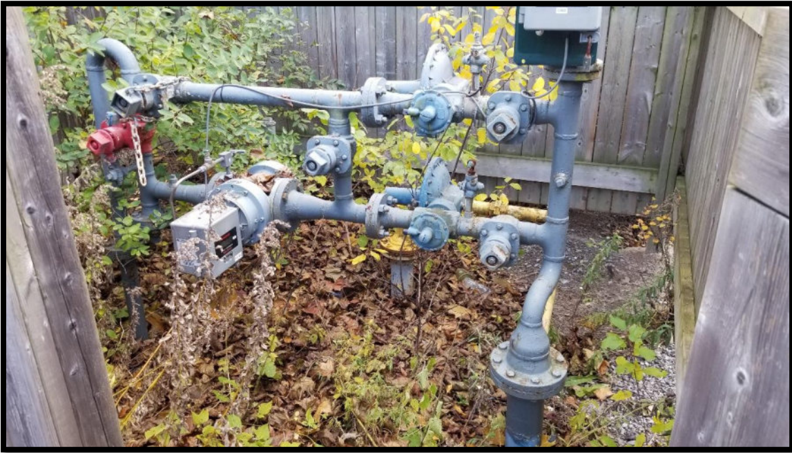
Photograph 7: Natural gas enclosure, observed between Buildings B and M. Site utilities are present underground, throughout the complex.
