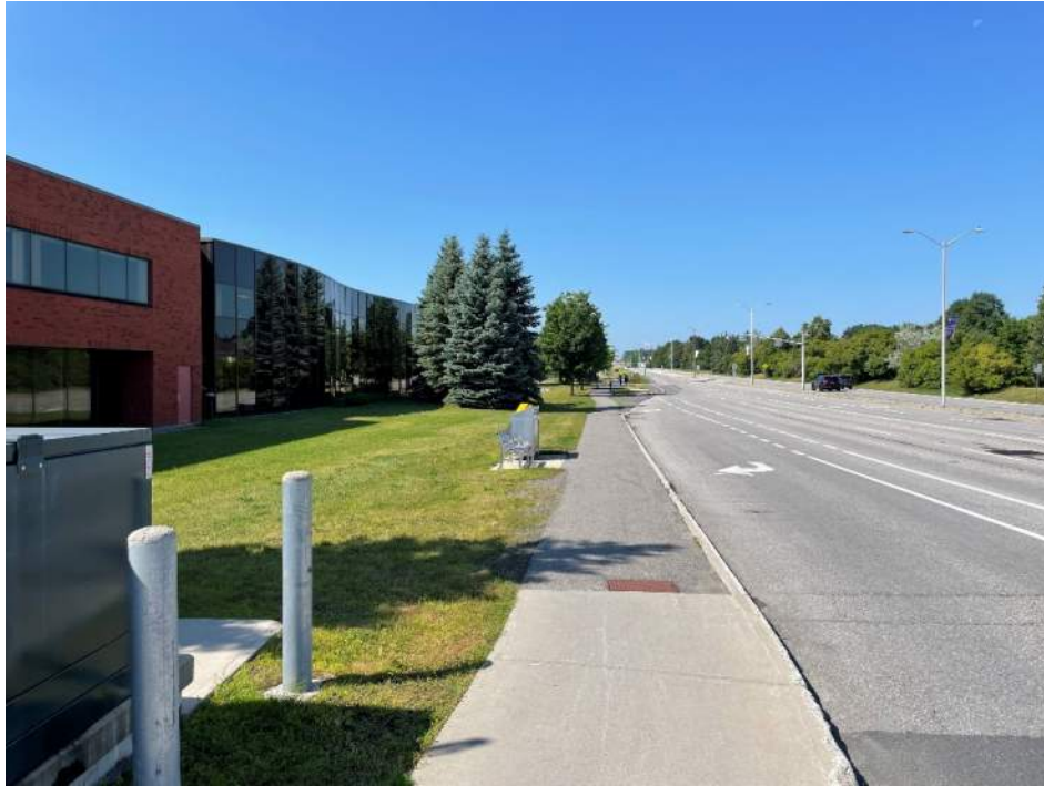
Photo 1: Northern corner of the phase one property looking southwest along property line. Northern most oil filled transformer in foreground on the left side of the photo.
