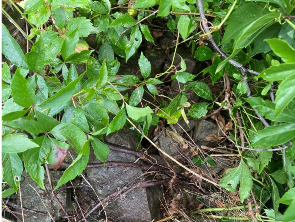
Photo 17: Broken rock fill observed on the phase one property at the corner of Hines Road.
