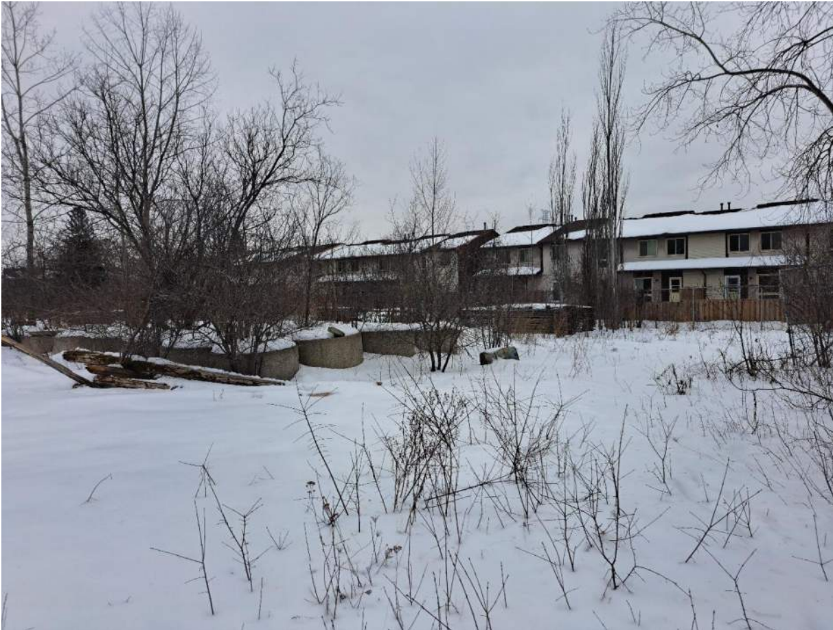
Photograph No. 8: Concrete and Wood Debris
