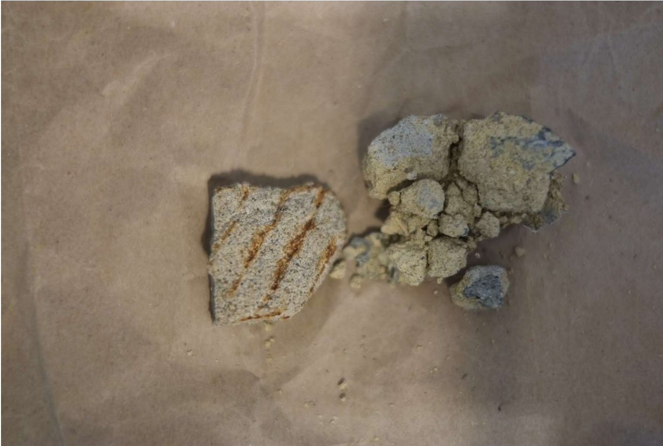
Fig. 3: Stucco substrate is crumbling and separating from rusty support wire mesh. Impossible to remove stucco panels without damaging them.
