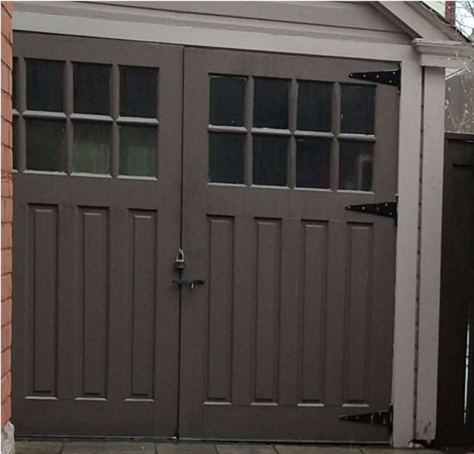
Fig. 21. Garage doors were replaced by then owner in the 1990's as original doors were finished. Doors swing sideways and cannot be opened during the winter months due to frost heave of the driveway in front of the garage. Doors were cut 2 inches last year to attempt to correct issue, but another 2 inches would need to be cut from the bottom so that they could swing open properly.
