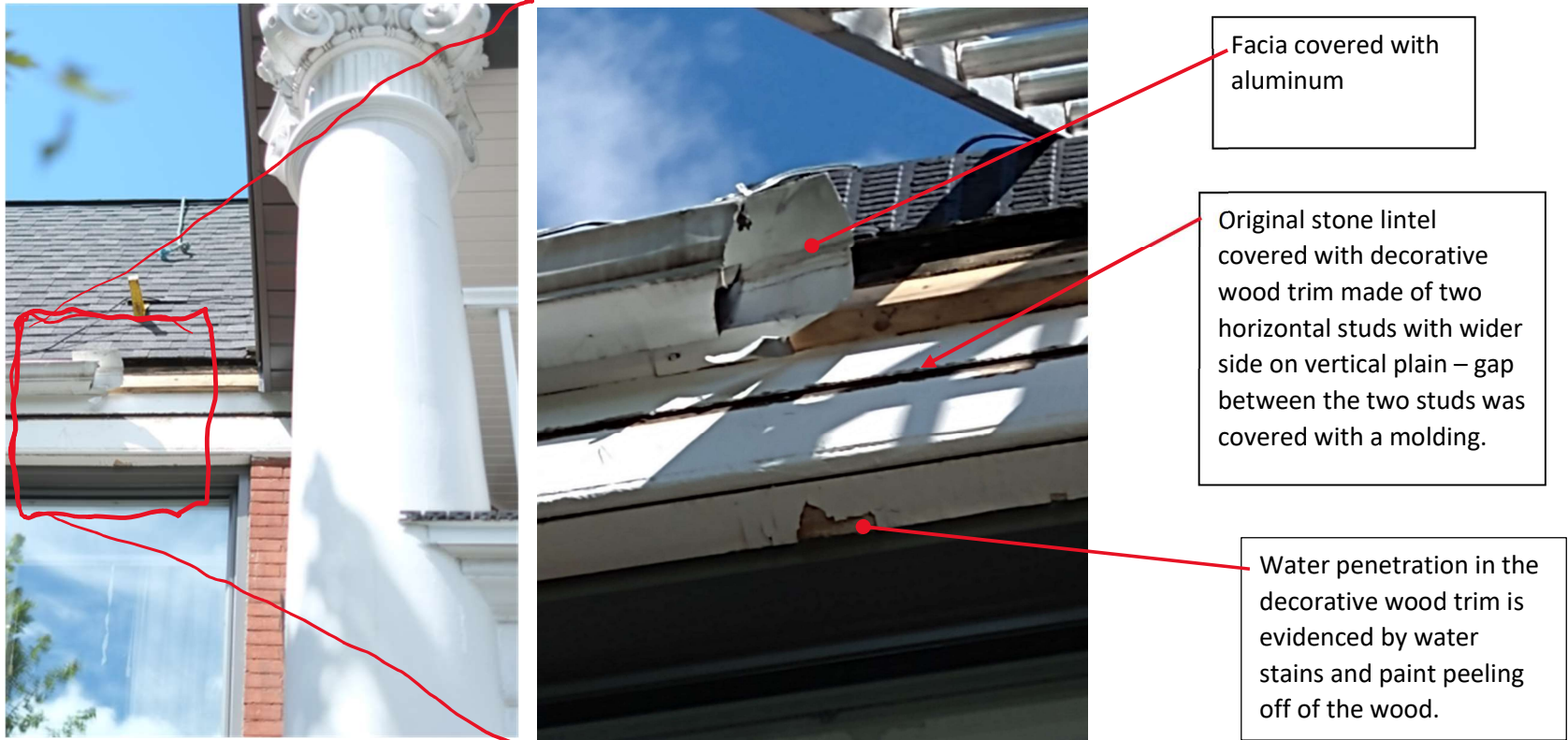
Fig. 8 and Fig. 9: Front of house – upper facia and decorative trim above 2 nd floor windows: Photo shows that facia was covered with aluminum. Rain gutter was also installed. Water penetration is evident. Long term concern is water damaged wood will attract infestation of insects such as carpenter ants.
