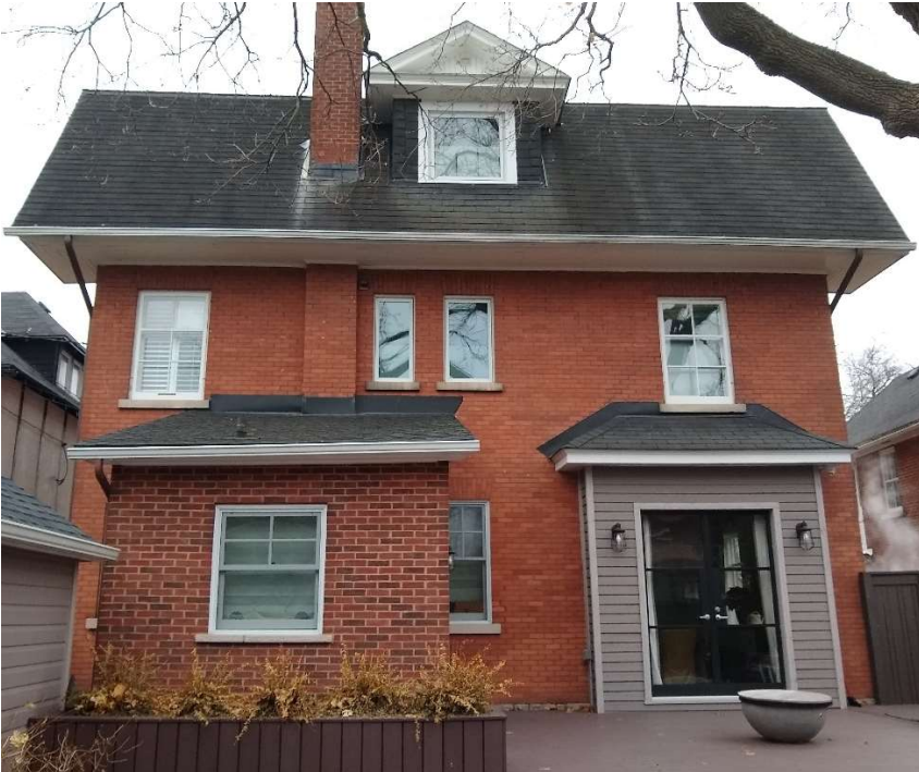
Fig. 17: Before. Asphalt shingles used on dormer
