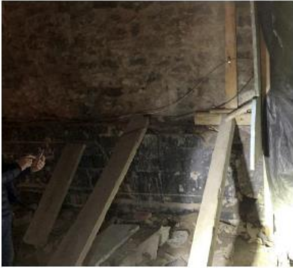
Figure 49: Deteriorated condition of the north foundation wall.
