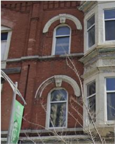
Figure 20: Missing arched metal lintel on west façade.
