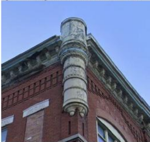
Figure 17: Peeling paint, open soffit, and general deteriorated condition of corner turret.
