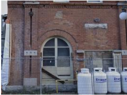
Figure 6: Brick efflorescence and debonded joints above the window on the north façade.
