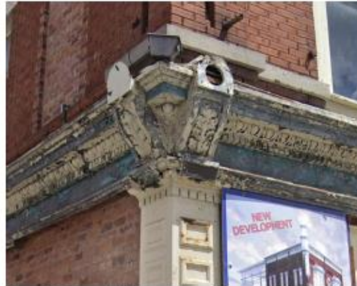
Figure 16: General deteriorated condition of first floor cornice.
