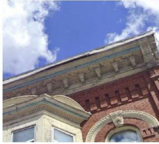
Figure 18: Separated fascia, deteriorated cornice and frieze.
