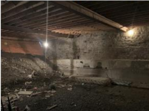
Figure 51: Backfilling at the previous east wall and voids in the south foundation wall.
