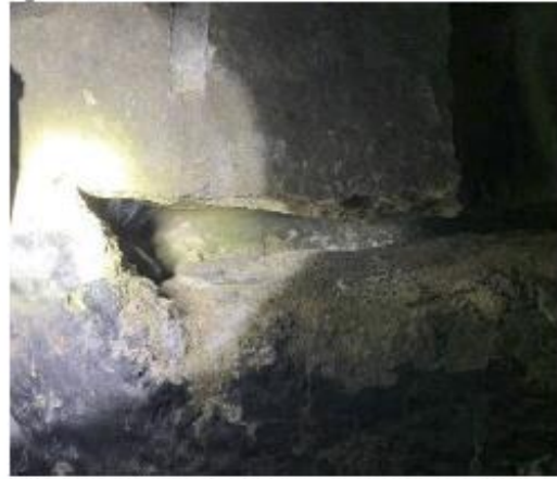
Figure 52: Deteriorated condition of mortar and voids in the stone foundation.
