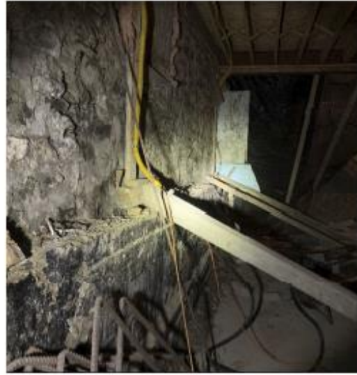
Figure 50: Cracks in the concrete foundation wall.
