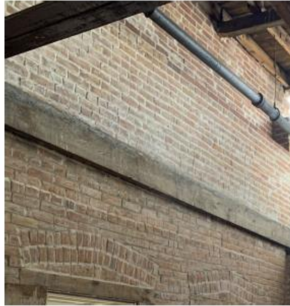
Figure 46: Deteriorated brick on interior of third floor with debonded wythes, frost damage, and surface damage.
