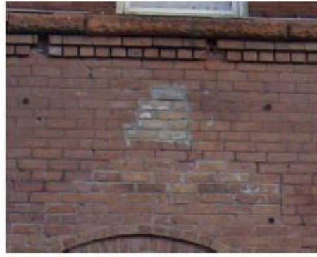
Figure 7: Incompatible previous repair above north façade door and deteriorated brick corbelling above.
