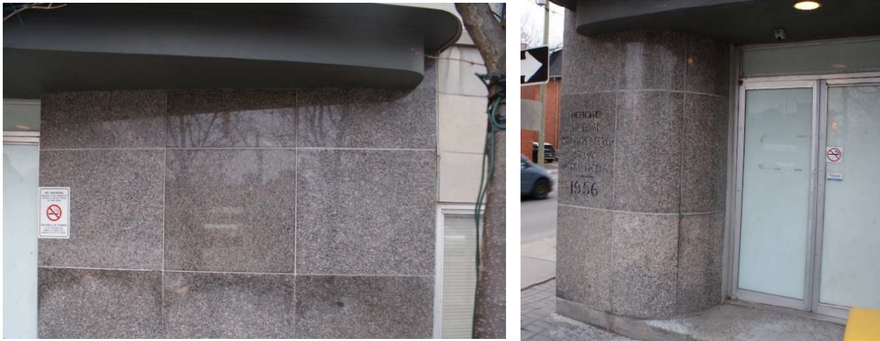
Figures 16 & 17: (6 -left) View of the introduced polished granite panels to the right of the Gilmour Street entrance. (7-right) View of the original polished granite panels. Source: Commonwealth 2023
