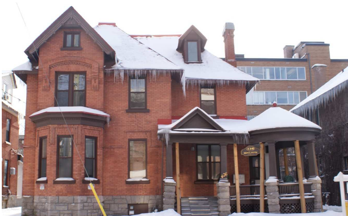
Figure 35: View of 436 MaClaren Street. The masonry piers supporting the porch have settled due to inadequate foundation depth. A detailed assessment of the condition of the porch is required. Guidelines from the CHCDP provide guidance for the conservation approach to the materials and assemblies. Source: Commonwealth 2023.
