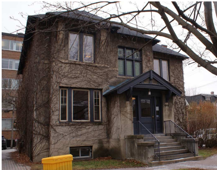
Figure 36: View of 444 MacLaren Street. The stuccoed exterior wall is covered in vines that should be removed before they have an adverse impact on the stucco finishes. Source: Commonwealth 2022
