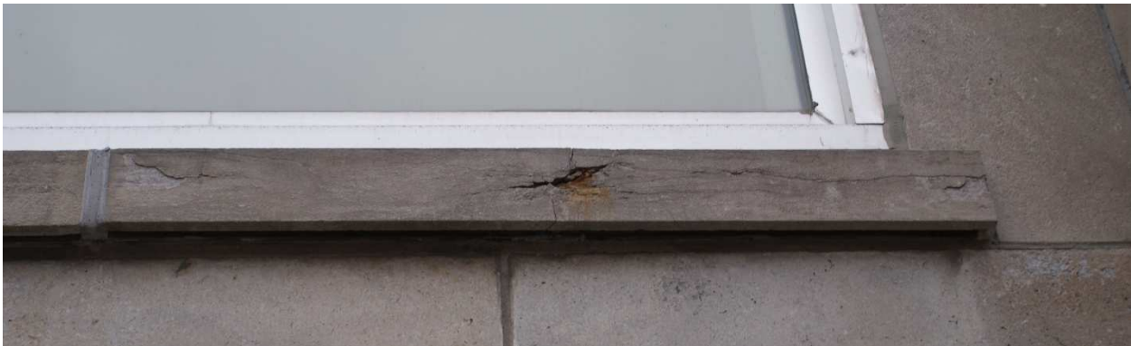
Figure 21: View of a deteriorated limestone windowsill. The cleavage planes within the limestone sills are evident where the sawn surface. The cleavages planes follow the layers of deposition of the sedimentary rock. Source: Commonwealth 2022.
