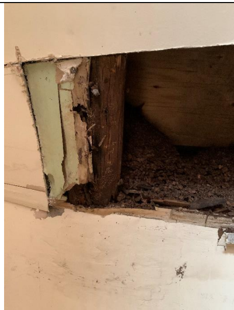
Photo 6: Third story north sloped roof; damage noted within roof and on roof joists [JCAL 2021]
