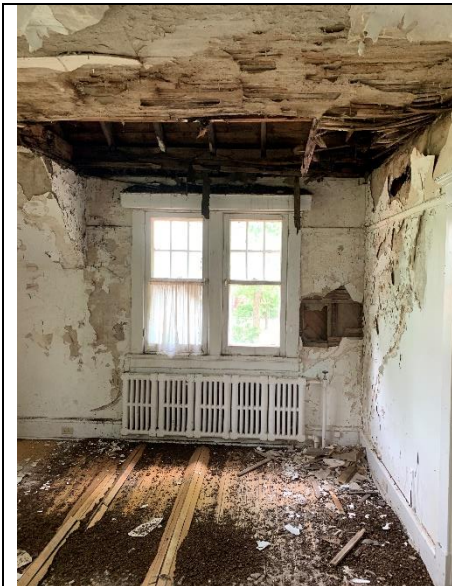
Photo 1: South second story wall overview, damages noted to floor, wall and ceiling finishes surrounding the area of significant water damage [JCAL 2021]
