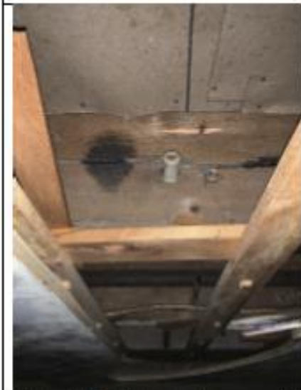
Photo 23: Mold noted on ground floor structure [JCAL 2021]
