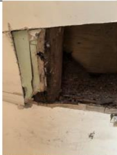
Photo 6: Third story north sloped roof; damage noted within roof and on roof joists [JCAL 2021]
