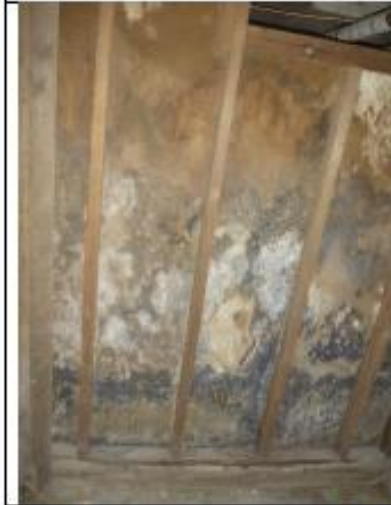
Photo 9: Interior basement wall typical condition with extensive mold. [JCAL 2021]
