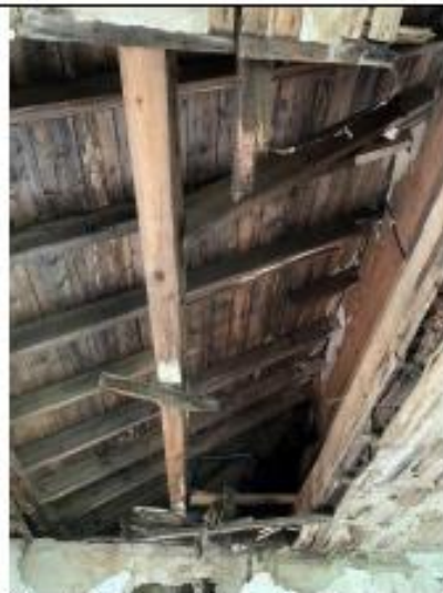
Photo 2: View into ceiling damage shown in photo 1- roof rafters decaying [JCAL 2021]
