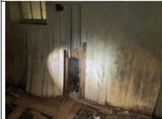
Photo 21: Typical extent of mold throughout basement [JCAL 2021]
