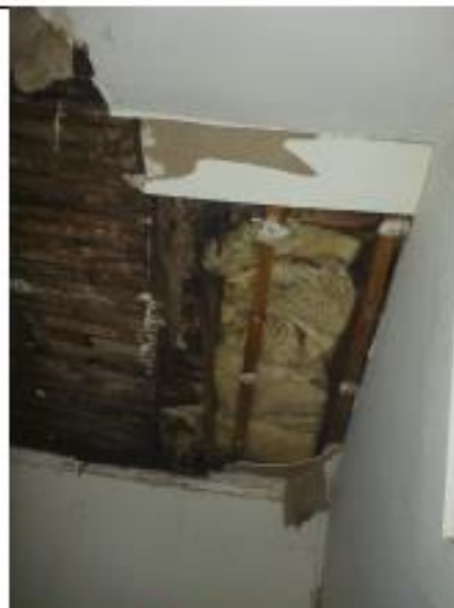
Photo 14: West room closet water damage and mold [JCAL 2021]
