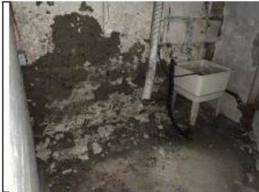
Photo 7: Concrete foundation damage and salt deposits [JCAL 2021]
