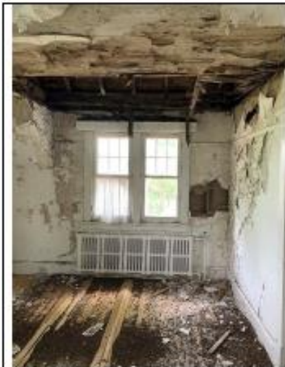
Photo 1: South second story wall overview, damages noted to floor, wall and ceiling finishes surrounding the area of significant water damage [JCAL 2021]
