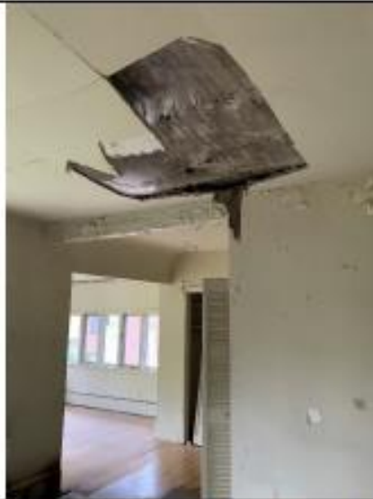
Photo 16: Second floor damage to ceiling finishes [JCAL 2021]
