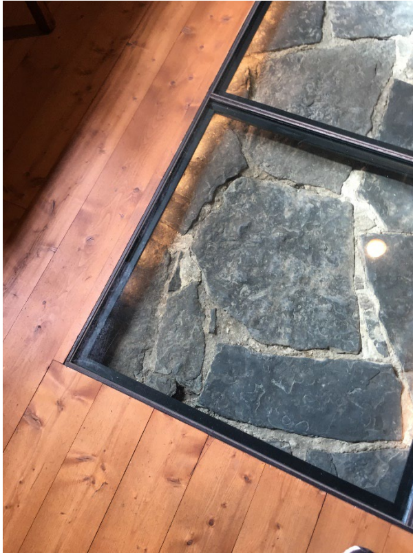
Figure 9 – New/ old connection detail - Le Monastère des Augustines, Quebec City (Photo: RMA+SH, 2021).
