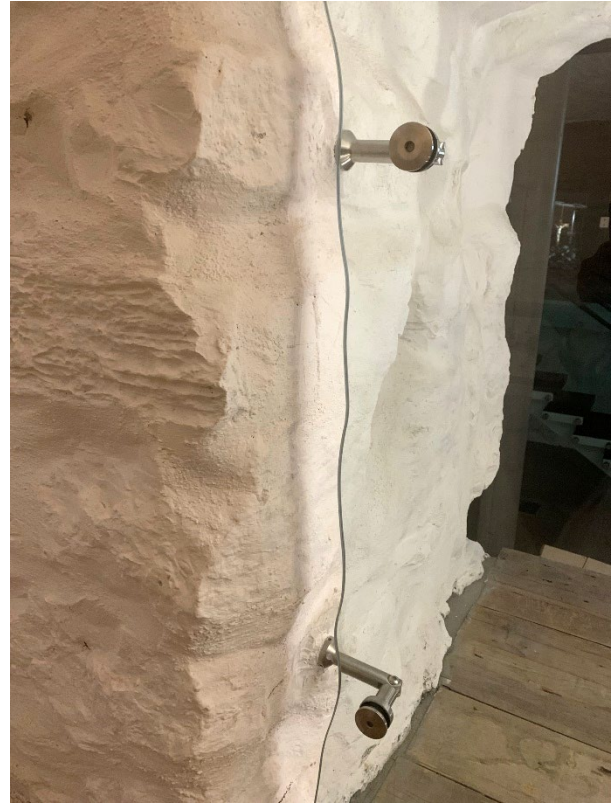
Figure 10 – New/ old connection detail - Le Monastère des Augustines, Quebec City (Photo: RMA+SH, 2021).
