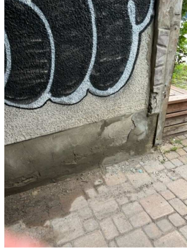
Photo 6: Cracking in back of veneer.
