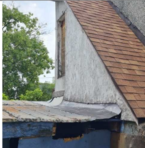
Photo 35: Corrosion of roof sheathing.
