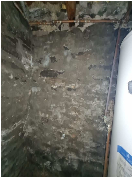
Photo 14: Previous Portland cement-based mortar application to interior surface.
