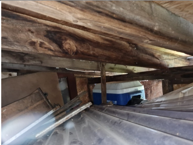
Photo 34: Dark wet staining on roof joists, indicative of rot.
