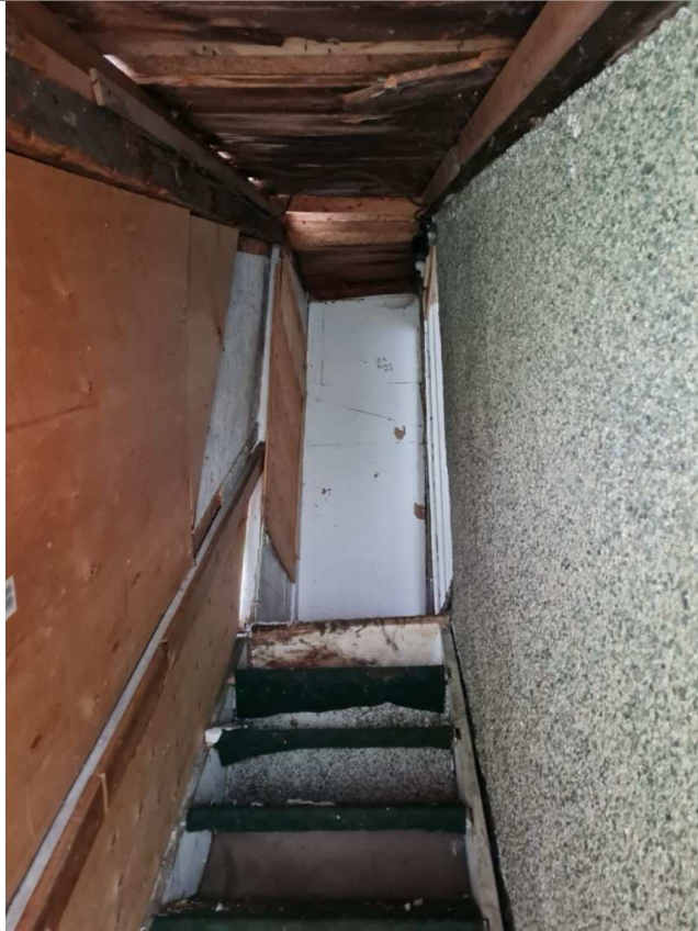
Photo 42: Timber appears weathered. Staircase is slanted.
