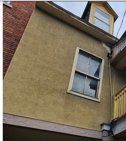
Photo 2: Front Stucco weathering & staining.
