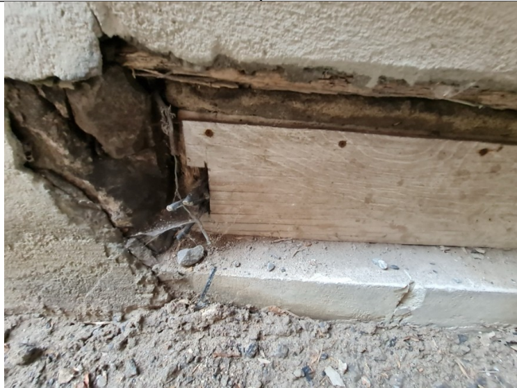
Photo 7: Foundation wall deterioration.
