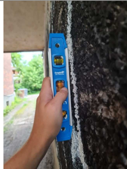
Photo 8: Laneway wall plumbness.
