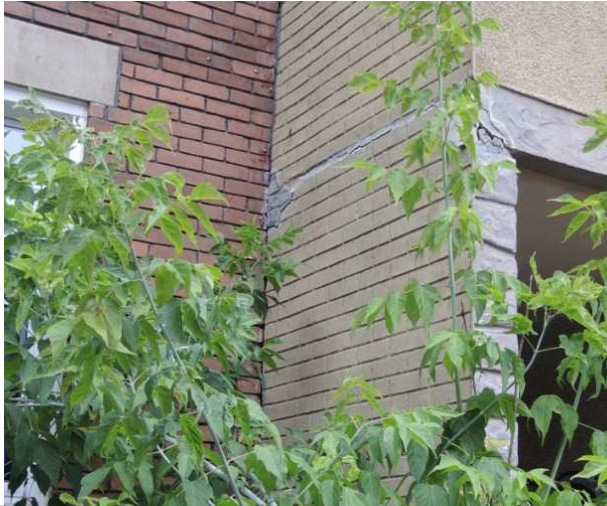
Photo 5: Horizontal cracking can be observed across the mortar in addition to cracking across the face of the bricks attached to the adjacent property. Cracking can also be observed at the corner above the laneway.
