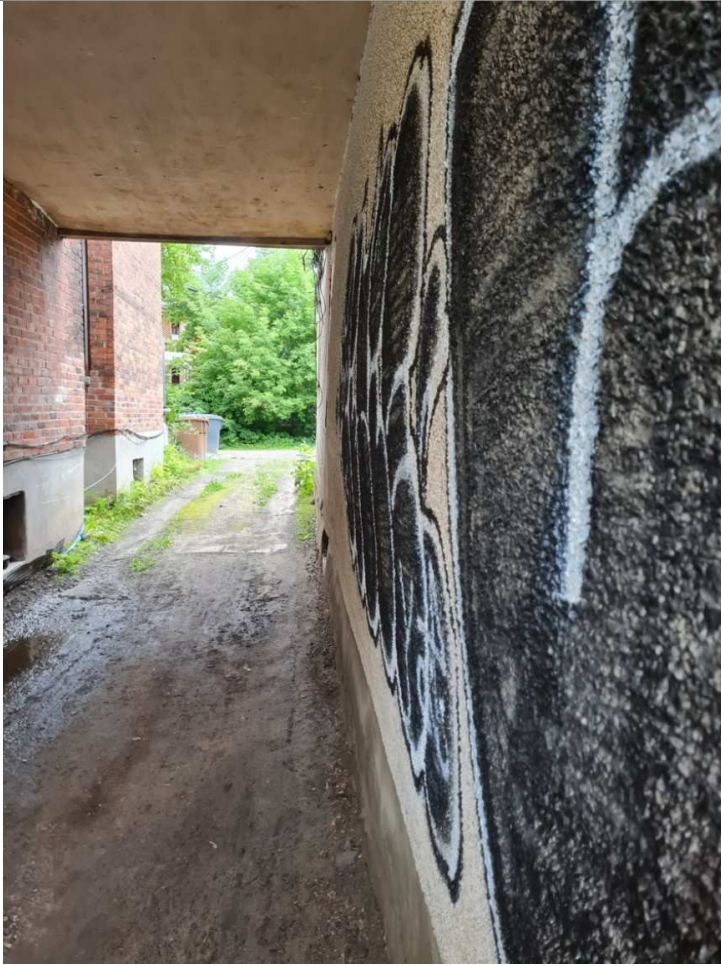
Photo 9: Bulging of laneway wall.
