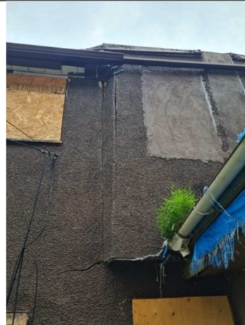
Photo 37: Stucco cracking and shifting visible on addition.
