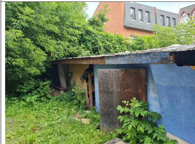
Photo 32: Shed is visibly settling and leaning.
