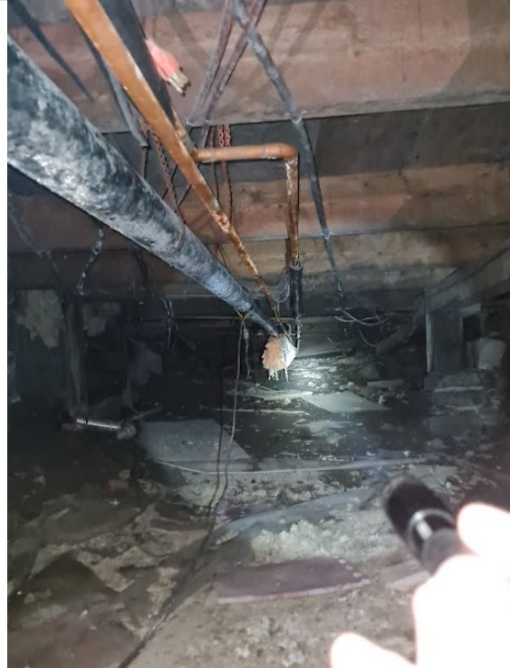
Photo 41: Crawlspace under rear addition shows partial collapse of the rear addition.
