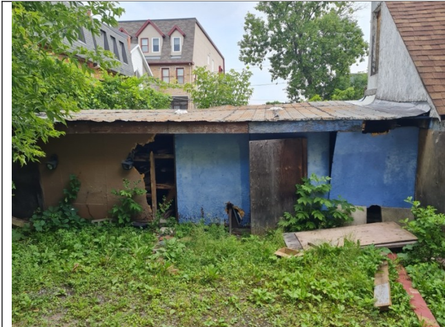
Photo 30: Certain pieces of wooden wall are broken/missing. Shed is leaning, roof slope is curved.
