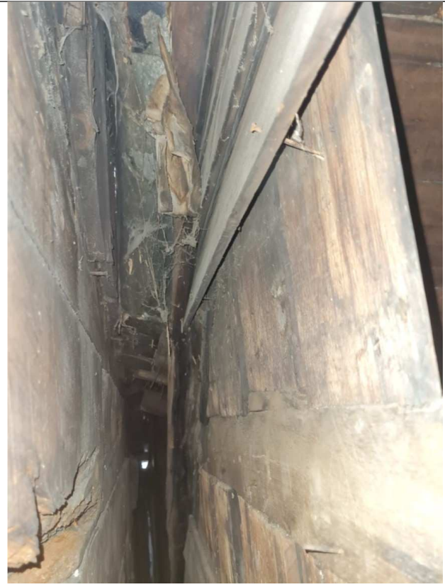
Photo 25: Inside of wall showing signs of decay along both structures. Daylight observed on all sides.
