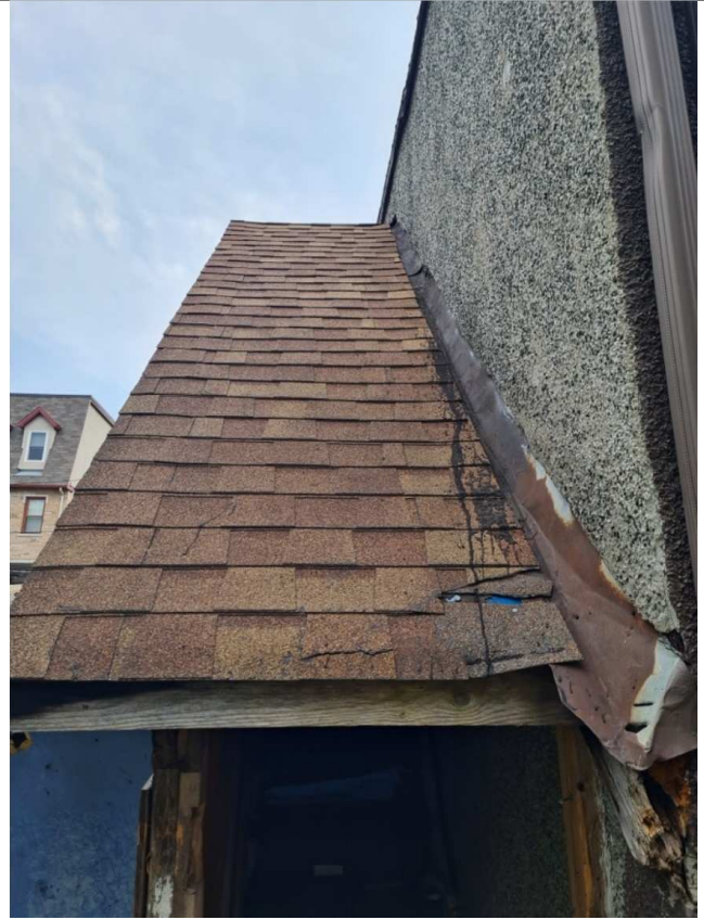
Photo 43: Poor flashing detail, corroding away.
