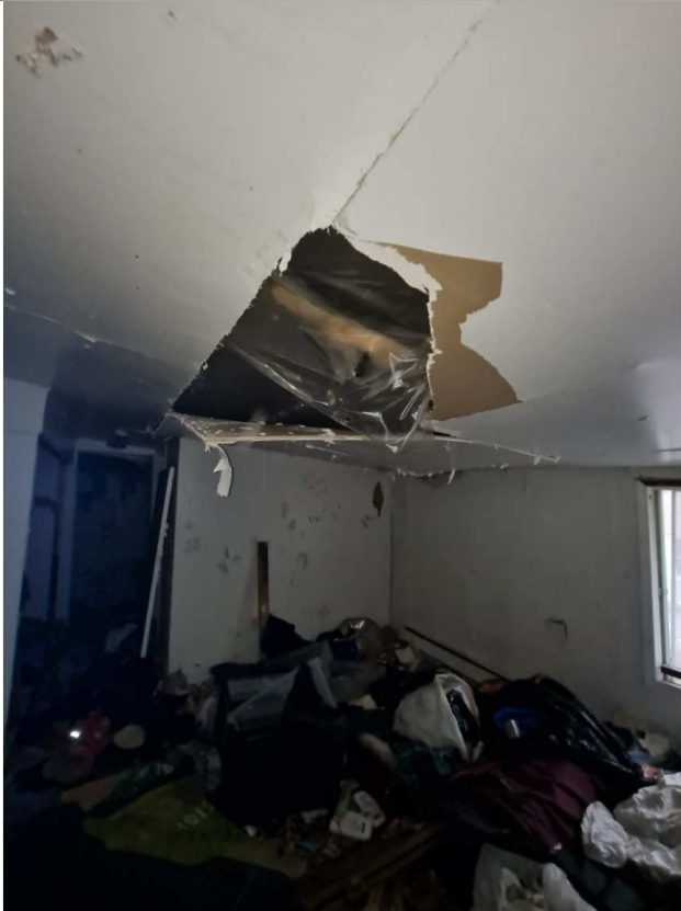
Photo 44: Ceiling is damaged and appears to be sagging.
