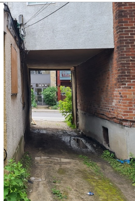
Photo 4: Laneway covering is slanted.
