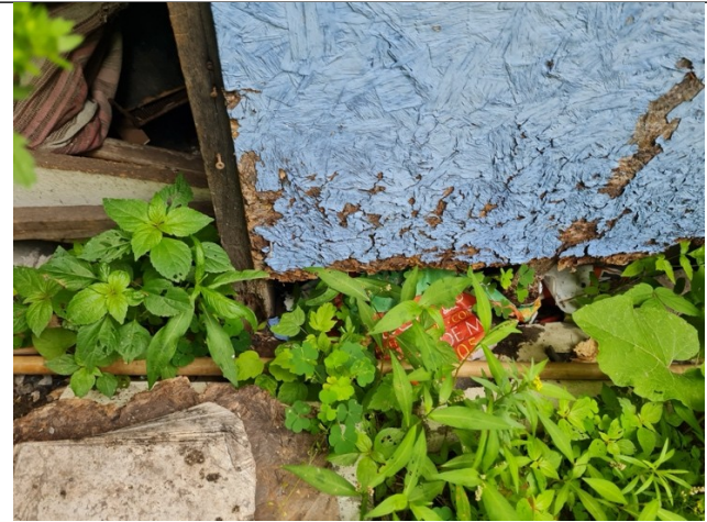
Photo 31: Shed lacks a foundation, bearing on water damaged areas. The paint is peeling, indicative of weathering of the wood.
