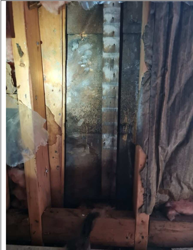
Photo 18: Exposed exterior wall showing signs of water damage on first floor at the front (South) wall of the building.
