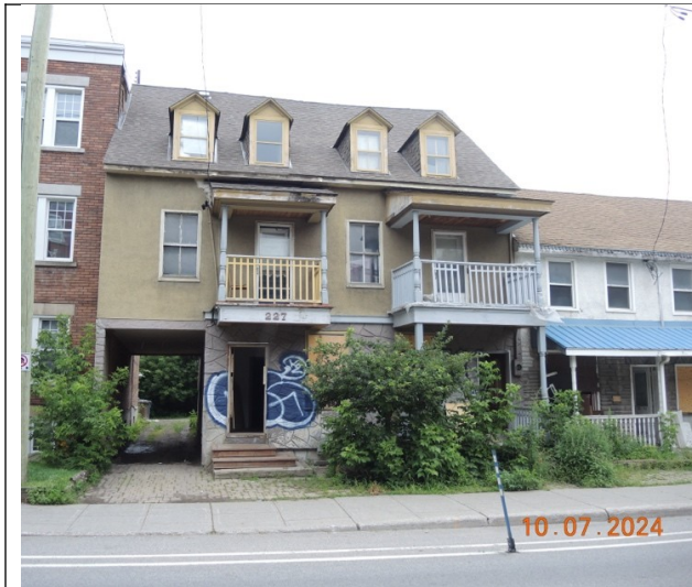
Photo 1: Paint peeling and weathering of wooden elements.
