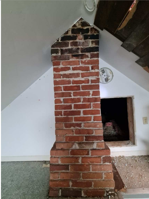
Photo 26: Chimney, with upper portion showing decay and moisture damage.
