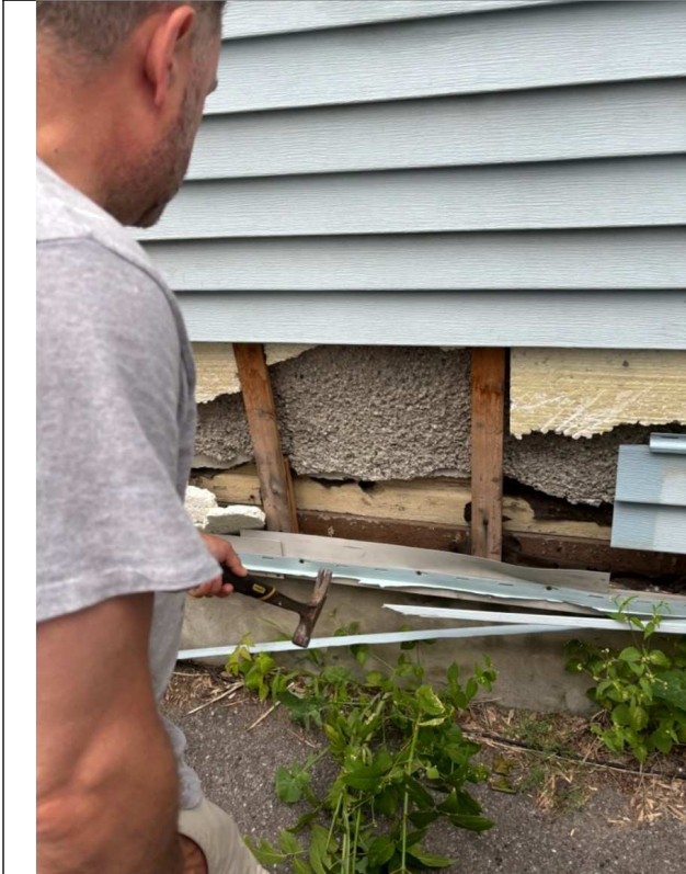
Photo 4: Siding has been applied on top of existing stucco and original wood siding.
