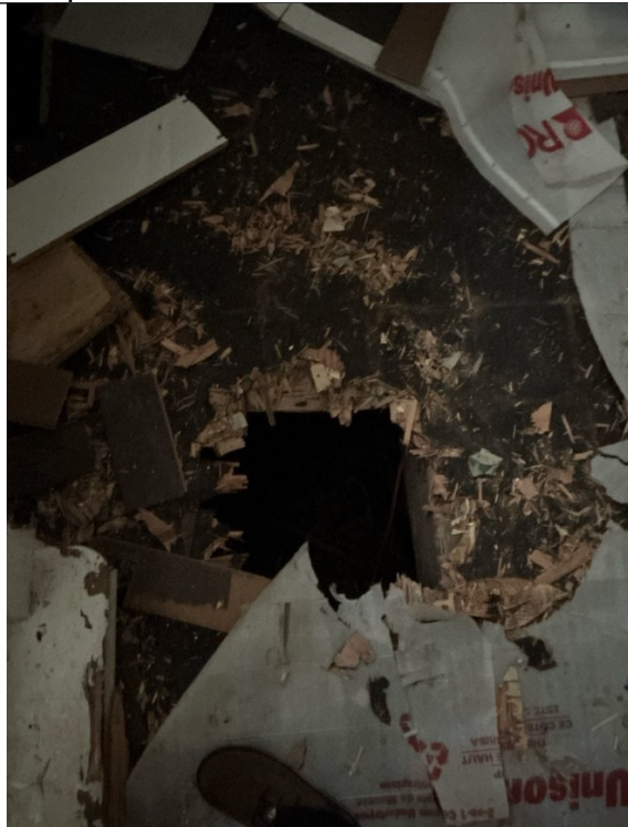
Photo 15: Hole in floor down to crawlspace. Rot is present.
