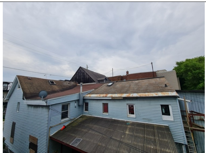
Photo 7: 231/233 St. Patrick St roof condition.
