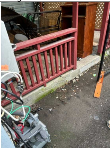
Photo 6: Cracking of the rear porch slab.
