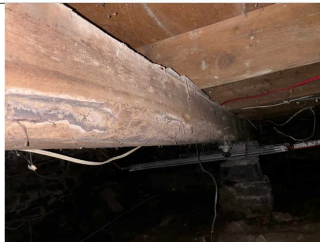
Photo 10: Decay on underside of main spine beam.
