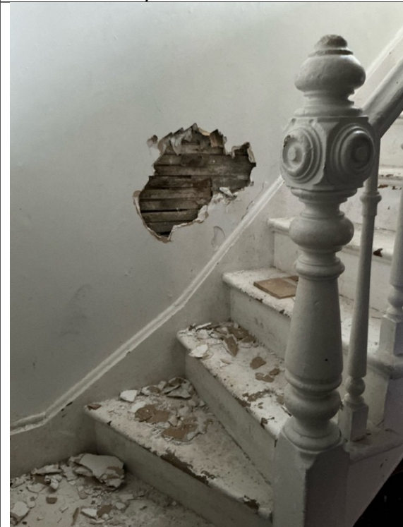
Photo 14: Exposed Lath showing signs of moisture damage.
