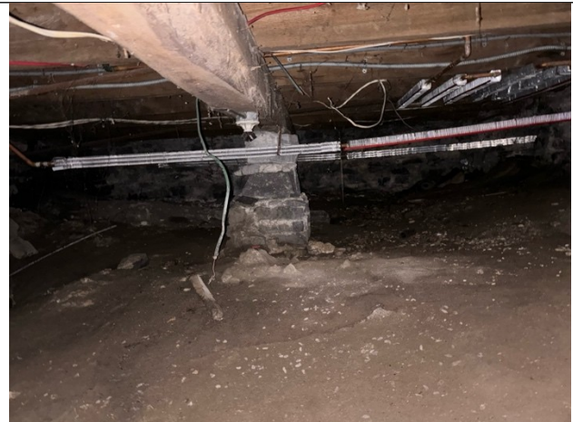
Photo 9: Deterioration of masonry pier.
