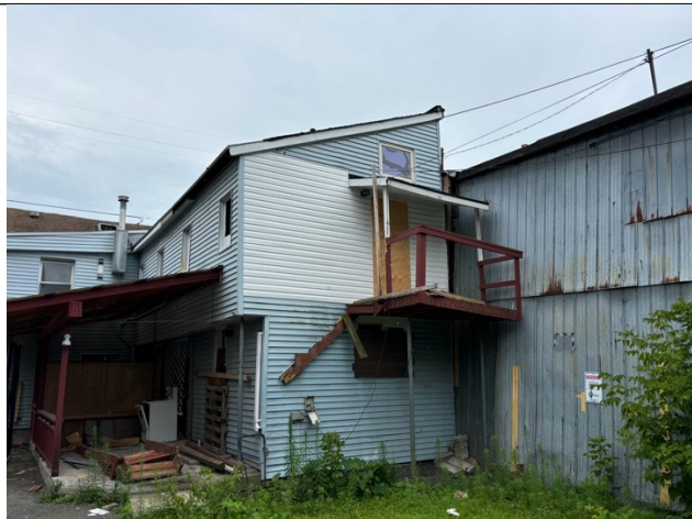
Photo 3: Elevated rear deck is leaning and is only supported by two jackposts.
