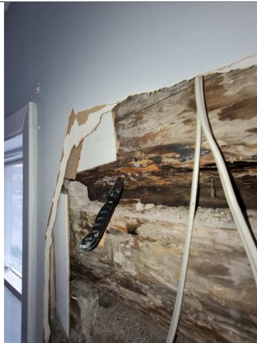
Photo 13: Field knife probe easily entered deep into exterior wall elements.
