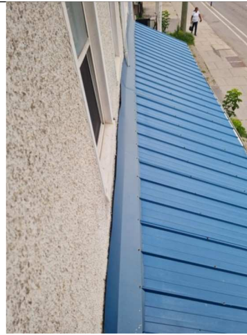
Photo 2: Flashing is not tied into stucco cladding and stucco is cracked along the interface.
