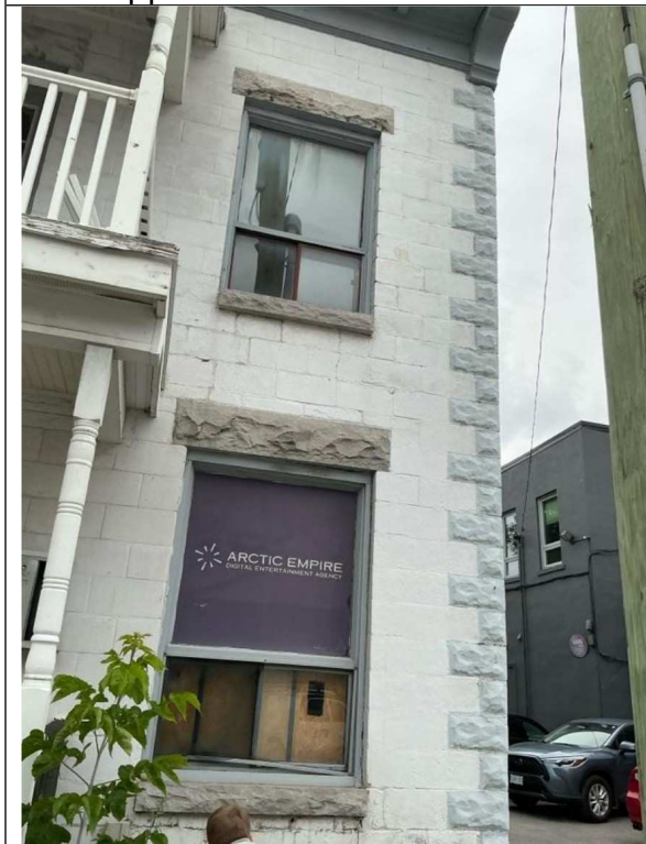
Photo 3: Weathering, vertical cracking and step cracking in faux-stone concrete veneer.
