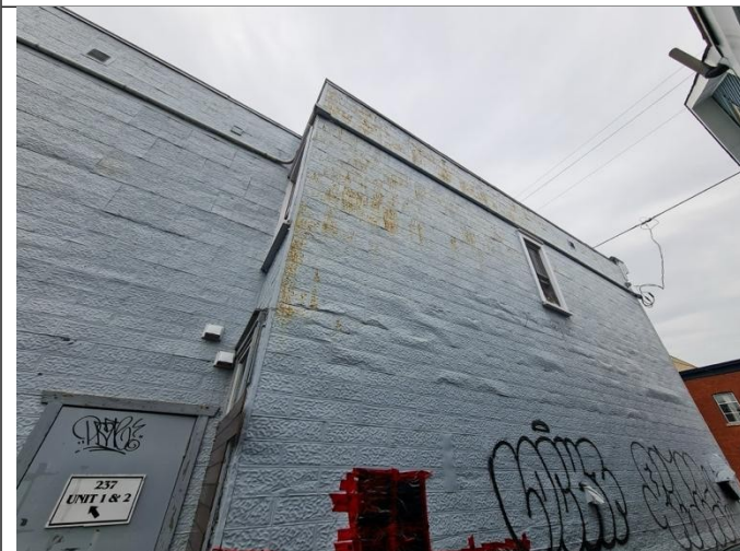
Photo 7: Bulging and peeling of existing cladding on West wall.
