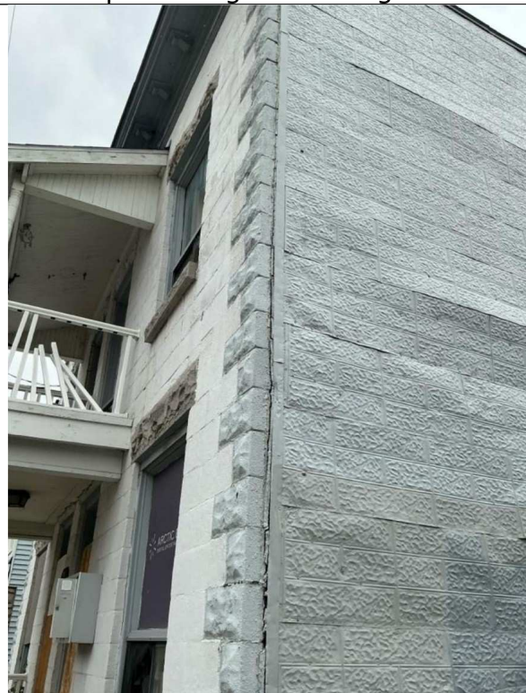
Photo 4: Nail applied tin panelling over timber wall (right) and Faux-stone concrete veneer detaching from underlying structure at South-East corner.
