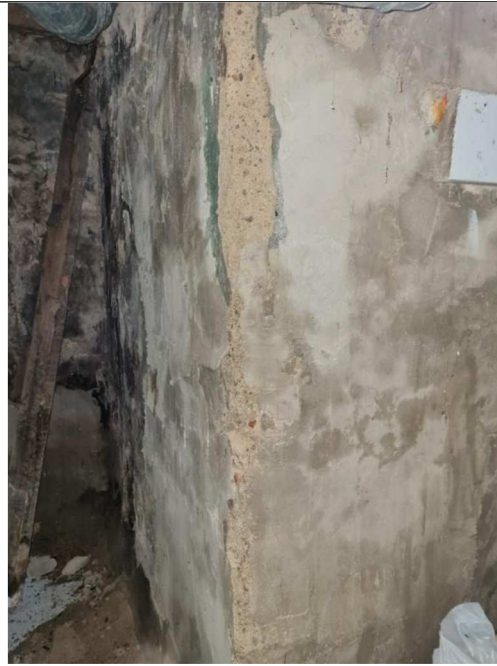
Photo 20: Deterioration of foundation wall.
