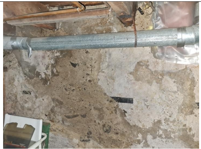
Photo 24: Severe scaling of the wall.
