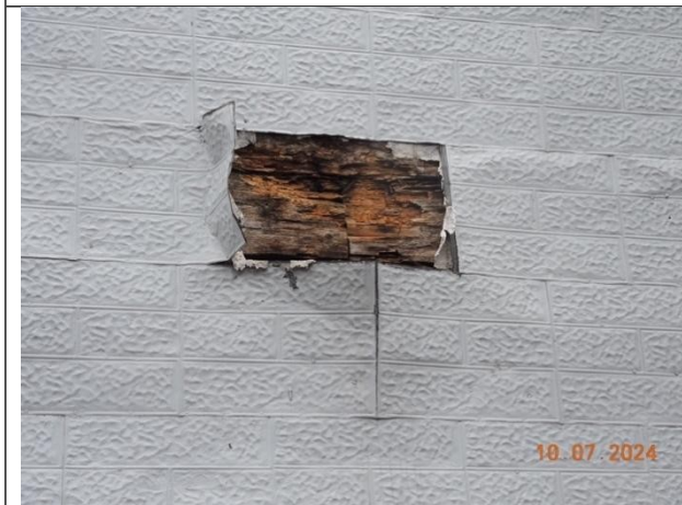
Photo 11: Advanced decay in exterior walls at opening in the cladding on East wall.
