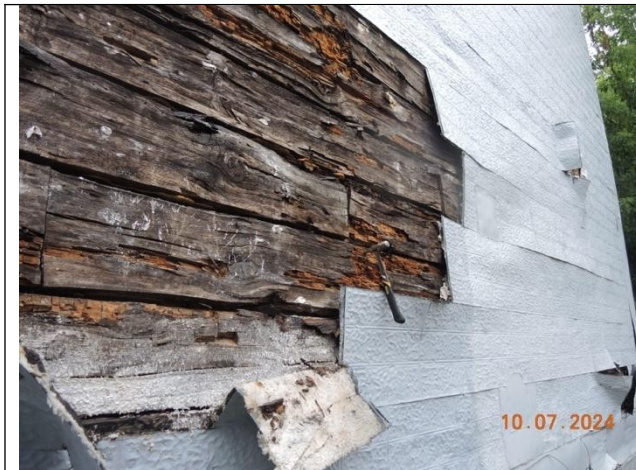
Photo 9: Advanced decay in exterior walls at opening in the cladding on East wall.
