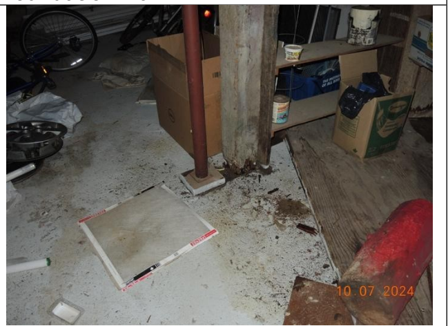
Photo 18: Base of main post rotting away.
