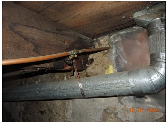
Photo 16: End of beam deteriorated due to rot. Beam has lost all connection to foundation wall.
