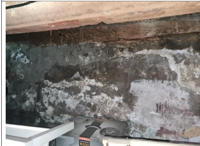
Photo 25: Efflorescence, discolouration & staining on the wall. Possible sulphate attack.
