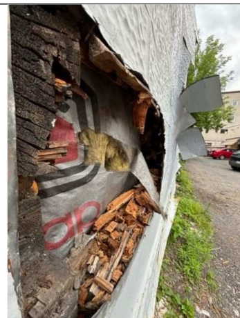
Photo 12: Remains of deteriorated wall are visible piling up at the base of opening in the East wall at the Southern edge.
