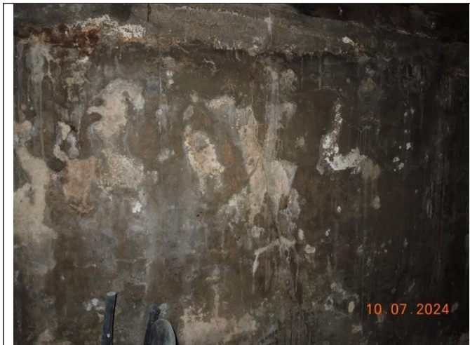
Photo 23: Crack and discolouration in foundation wall.
