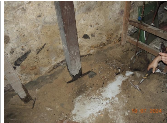
Photo 15: Sand build-up at base of wall due to deterioration.
