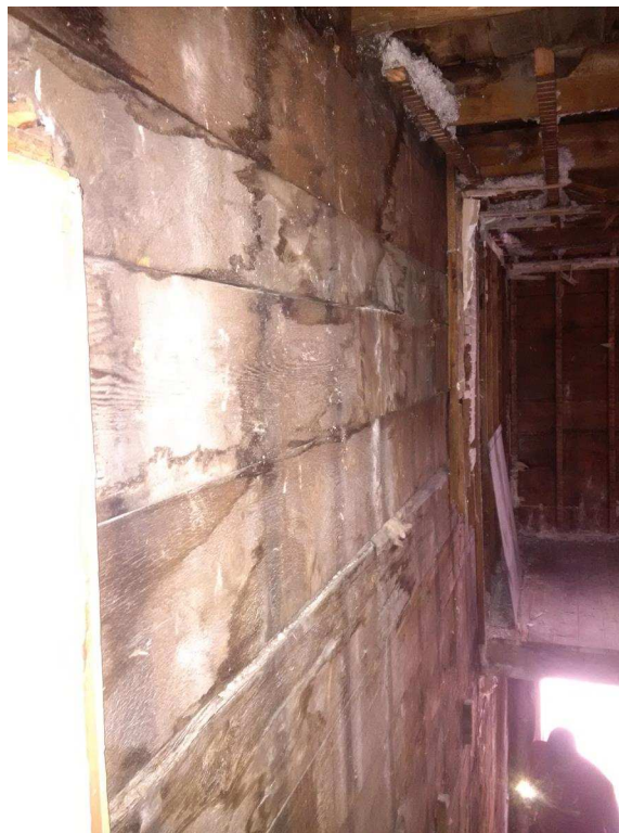
Photo Seven – Out of Plumb Wall/Water Infiltration
