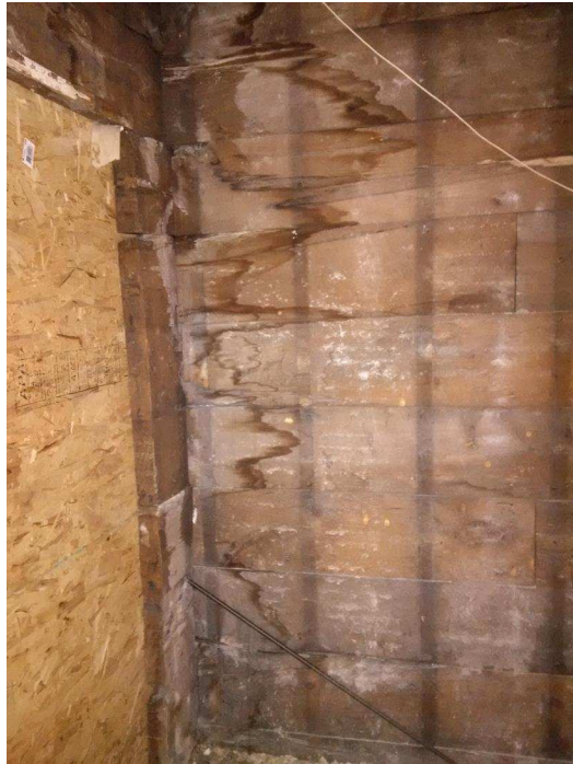
Photo One – Moisture Penetration
