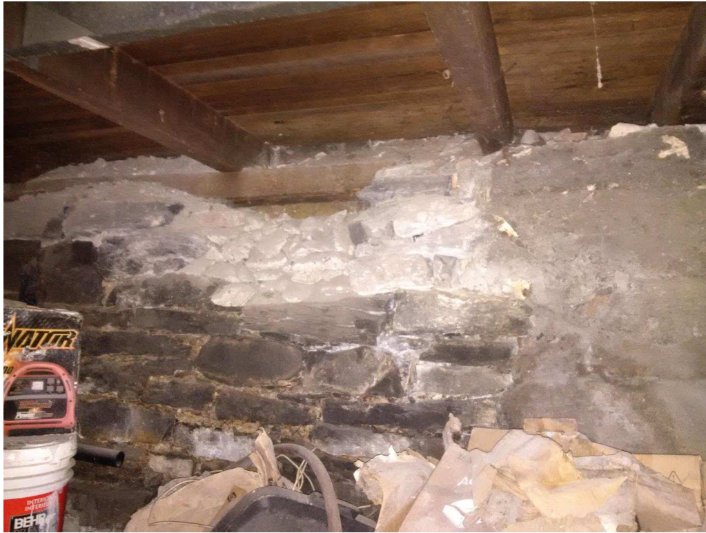
Photo Three – Dry Rot on Wood Framing
