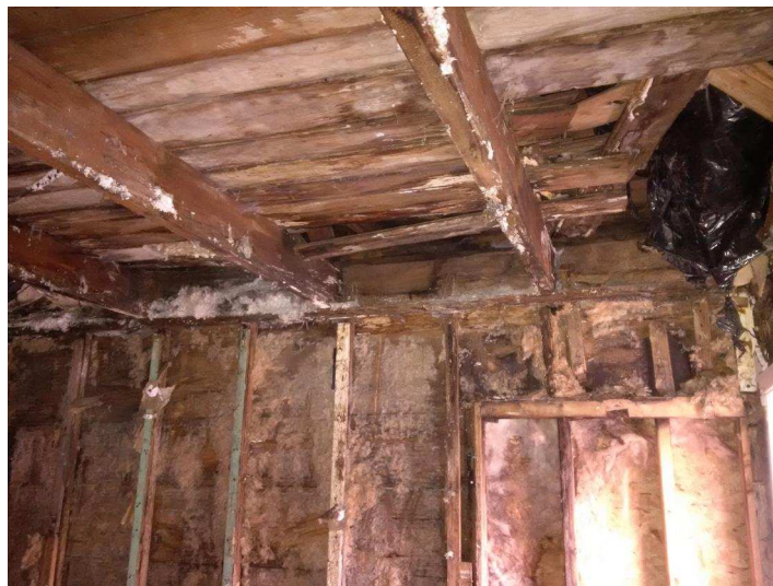
Photo Two – Water Damaged Roof Framing and Rot
