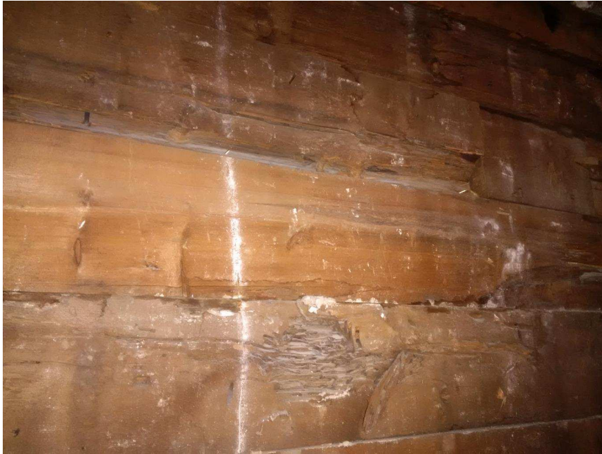
Photo Six – Carpenter Ant Damage
