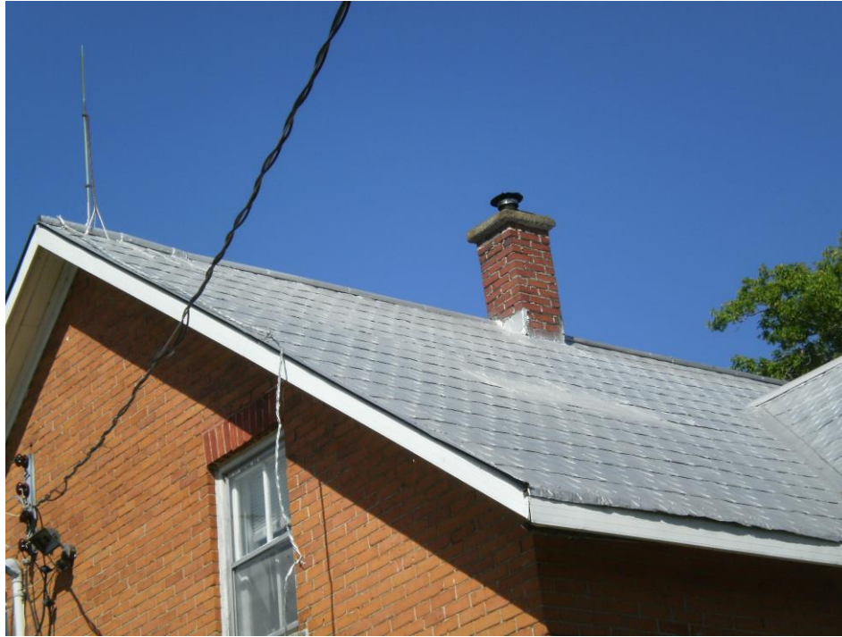
Photo 25 – Chimney is vented on the farmhouse in the northeast portion of the site west of Carp Road (June 10 th , 2018)
