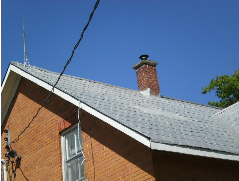
Photo 25 – Chimney is vented on the farmhouse in the northeast portion of the site west of Carp Road (June 10 th , 2018)
